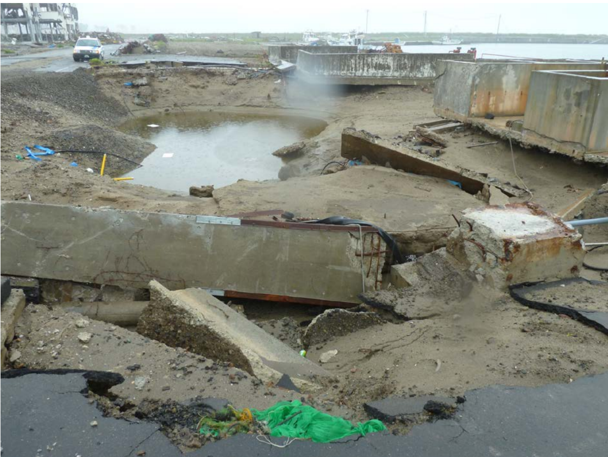
Figure 17 Bottom: scour, and collapsed reinforced concrete columns of the wharf and associated buildings at Yuriage, Miyagi, Japan, in the Great East Japan tsunami. Source: S. Fraser. Top: washout of some untied concrete tiles at Coquimbo wharf in the 2015 Chile tsunami (Horspool, et al., 2016).
