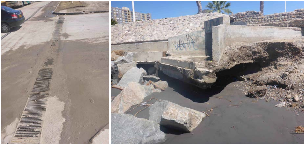
Figure 27 Left: Stormwater drain blocked by silt and sand in Coquimbo, Chile during the 2015 Chile tsunami. Right: Culvert/outfall at the coast in Coquimbo that was eroded during the 2015 Chile tsunami (Horspool et al., 2016).
