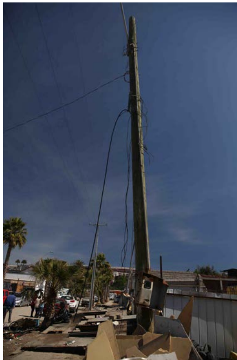
Figure 41 Example of damage to overhead lines in Coquimbo during the 2015 Chile tsunami (Horspool et al., 2016).
