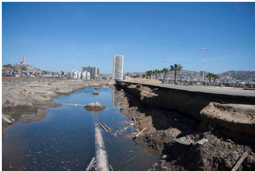
Figure 22 Top: Severed water main where it crosses a bridge in Coquimbo, Chile caused by erosion of the abutment. Bottom: severe scouring that exposed the same water main and caused it to float to the surface. (Horspool et al, 2016).
