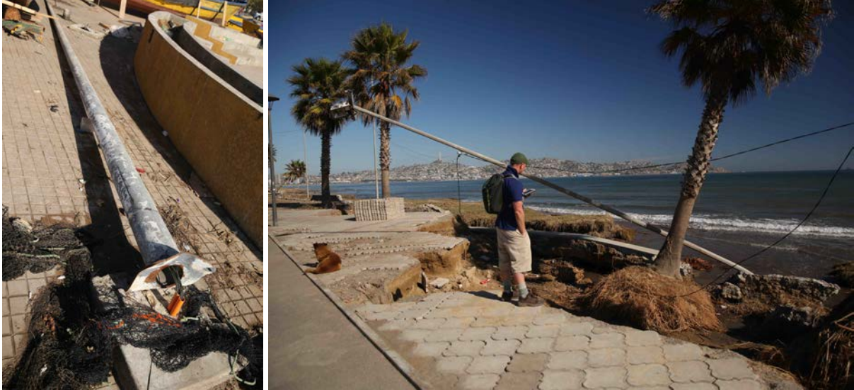
Figure 40 Example of damage to utility poles by shearing due to lateral forces or debris strike (left) and scouring of base (right) in Coquimbo during the 2015 Chile tsunami (Horspool et al., 2016).
