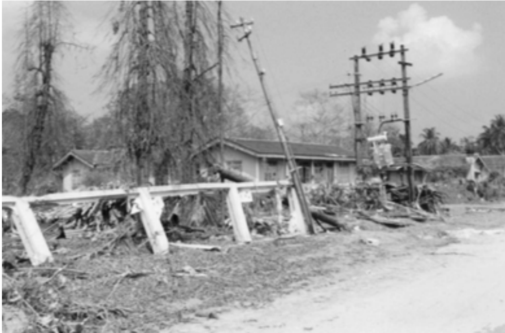
Figure 39 Example of damage to utility poles in Sri Lanka. In this example the poles have been moderately damaged and the tsunami inundated above the height of the pole mounted transformer, which later needed replacement. This would correspond to Damage State 1. (Source: Tang, 2006)
