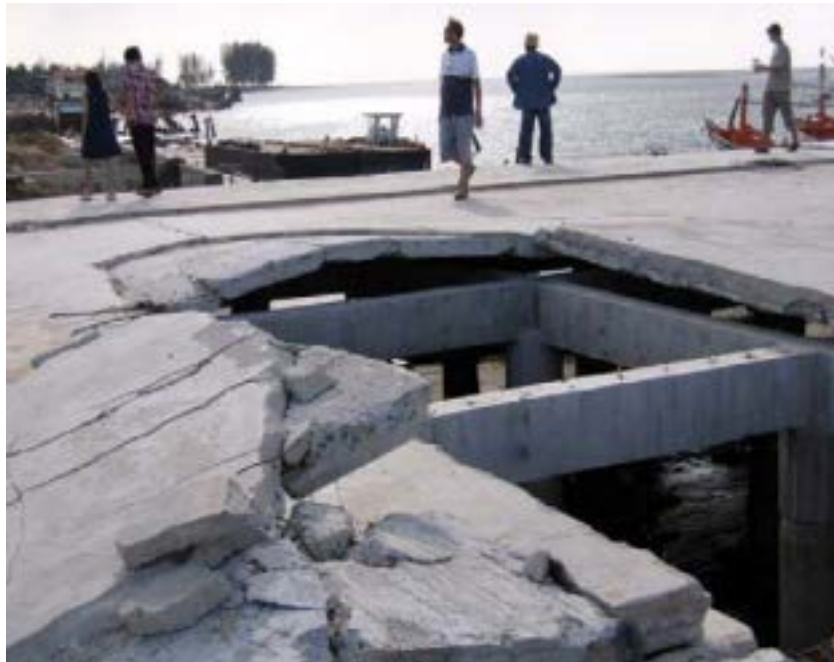
Figure 20 Damage to a wharf deck in Thailand from vertical buoyancy forces. Source: PARI, 2009.
