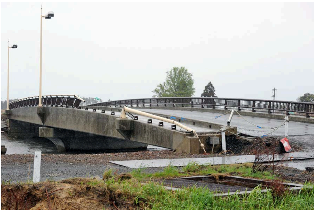
Figure 9 Bridge in Japan with minor-moderate damage of the superstructure and some minor scouring in the foreground. Source: Structural Engineers Association of Washington.
