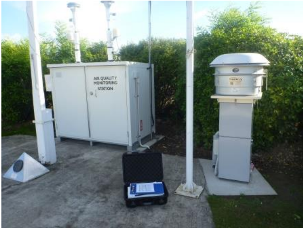
Figure 2.5: PM 10 monitor at the Redwoodtown - Bowling Club air quality monitoring site.
