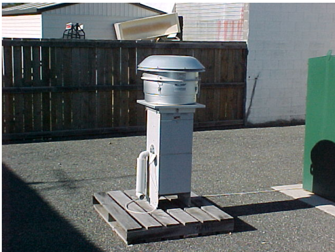
Figure 2.3: PM 10 monitor at the MRR air monitoring site
