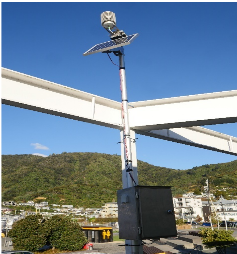
Figure 2-3: Air quality system at the Picton foreshore site.
