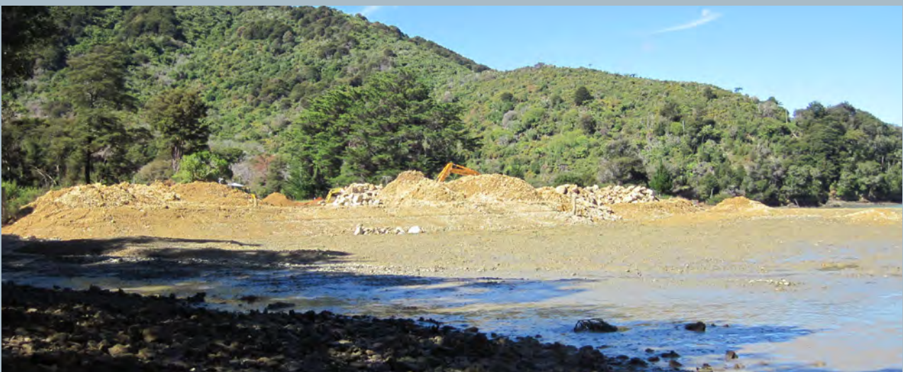
Marina development involving sediment scraping (see also above right photo) and reclamation.
