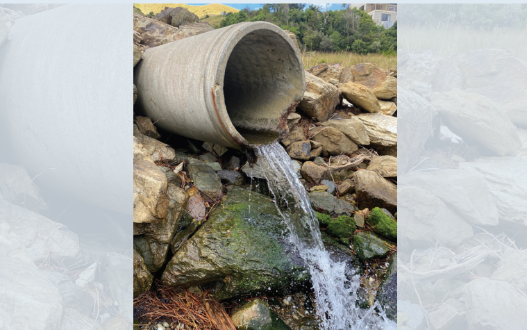
The above culvert has been installed very poorly. The edge is perched which results in no possible fish passage into the upper catchment.
