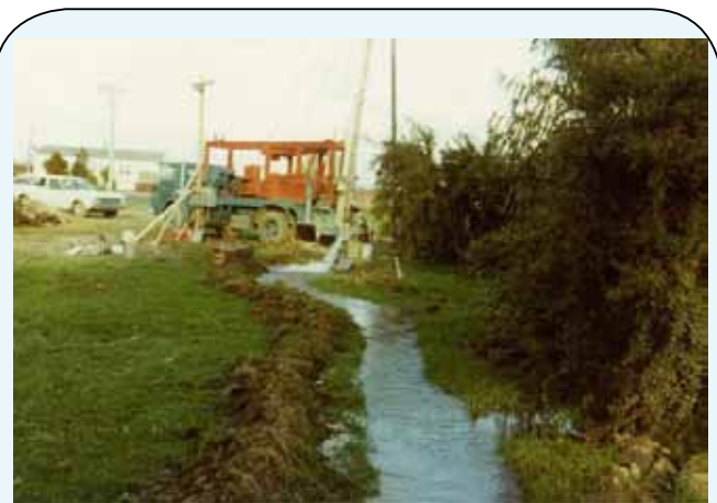
Figure 10.16: Test discharge water being disposed of at RNZAF Base Woodbourne in the early 1980s. A lined trench has been excavated to allow water to be directed away without infiltrating back to groundwater.
