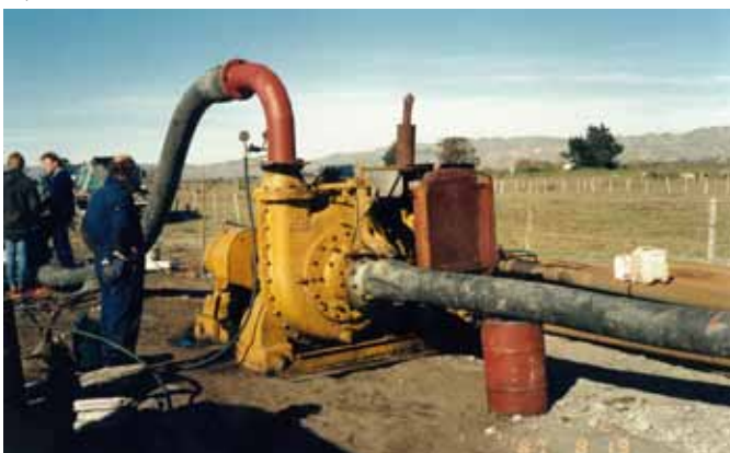
Figure 10.1: A very large surface mounted pump being used to test the Bar test well (1733) during a 72 hour test in 1987
