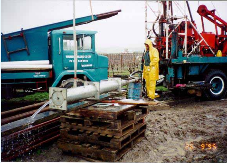
Figure 10.14: A single flow meter was sufficient for the small test rate used to evaluate the very low yielding Deep Wairau Aquifer involving the exploratory bore 2917 in September 1995. The person standing in the foreground is Mr C. Woodford, owner of Waimea Drilling Company Ltd. The rain which fell is less important when testing deep wells such as this where water bearing layers are several hundreds of metres below the surface.
