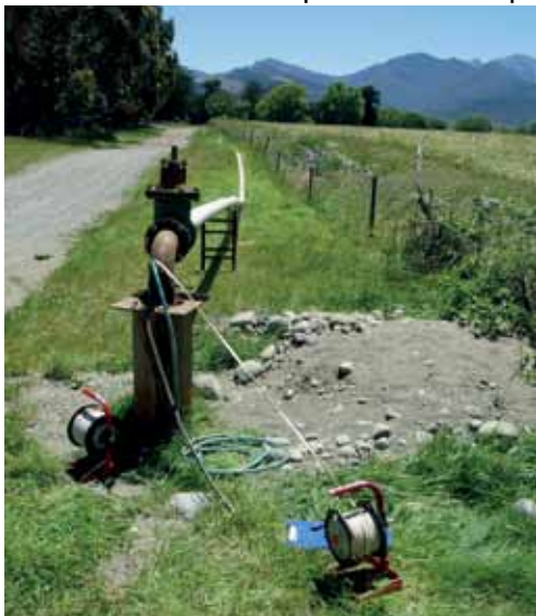
Figure 10.15: Discharged test water being piped north along Mill Road at Wairau Valley to Mill Stream during the December 2006 MDC test.
