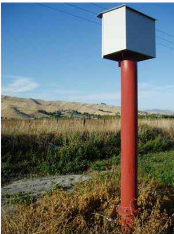
Figure 24.8: Extended well casing on MDC monitoring well 4402
