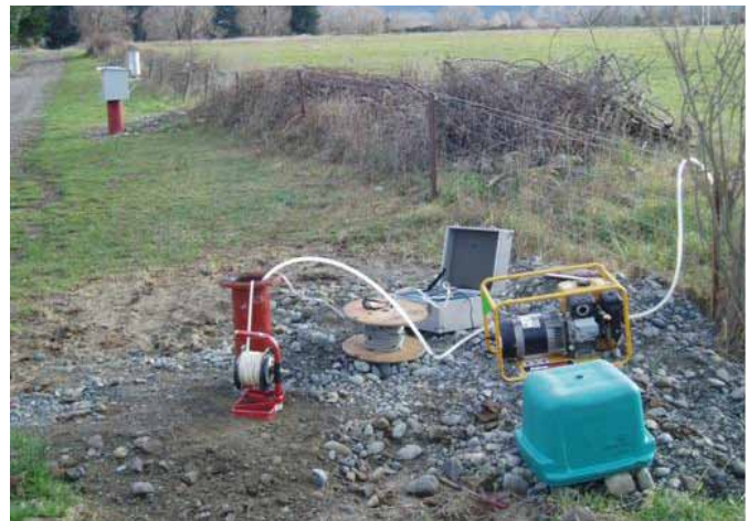
Figure 33.13: MDC Wairau Valley monitoring wells
