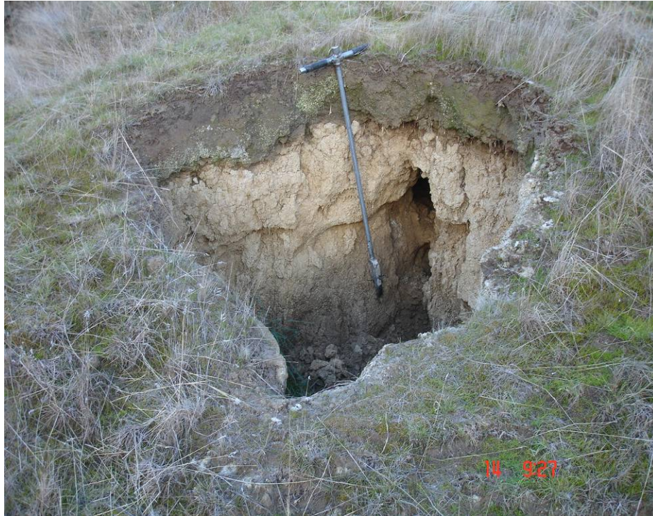
Figure 34. Roof collapse into an under-runner in a Wither hill soil.
