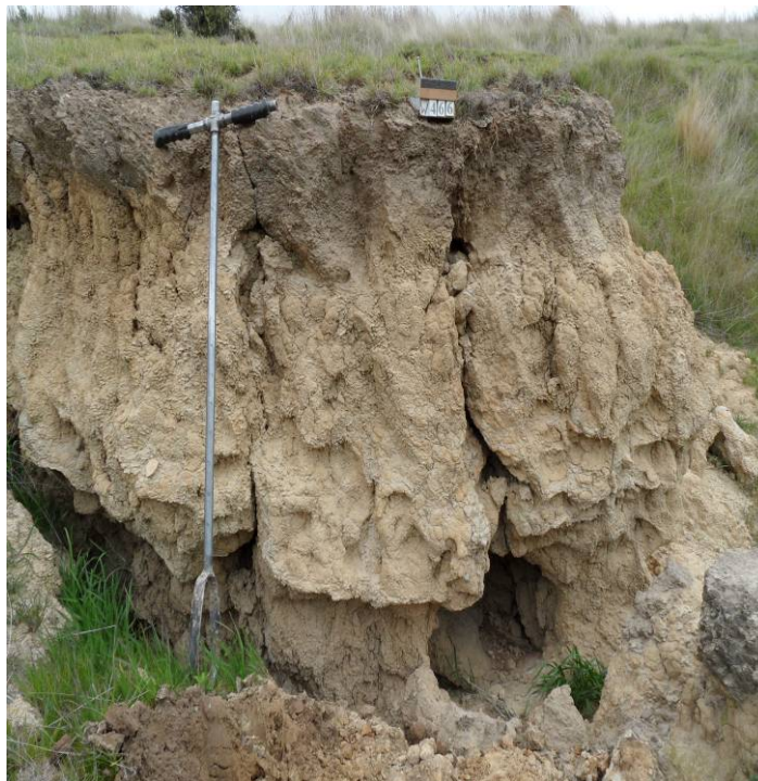
Figure 31. Soil cracks extending from the surface to the deep subsoil where tunnels have formed in the underlying highly dispersive material. Many existing cracks have probably formed due to instability caused by undercutting.
