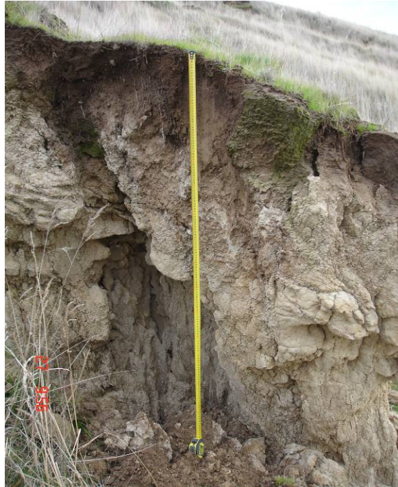
Figure 32. Enlargement of a subsurface cavern below a conduit above with partial collapse of the fragic horizon.
