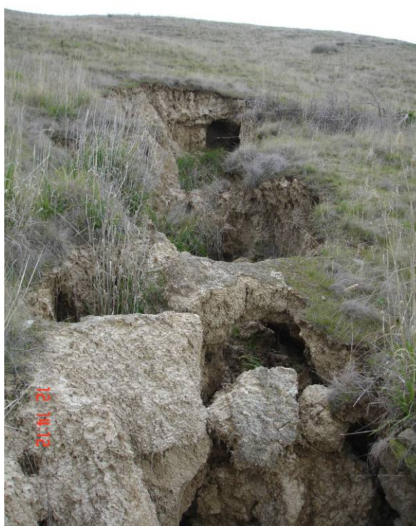
Figure 49. An actively eroding under-runner in Vernon soils with a partly collapsed roof and beginning to form a continuous gully.
