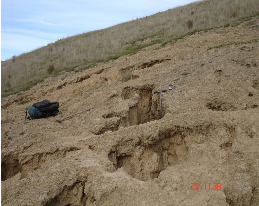
Figure 52. Sheet erosion and roof collapse into under-runners in Vernon hill soils.
