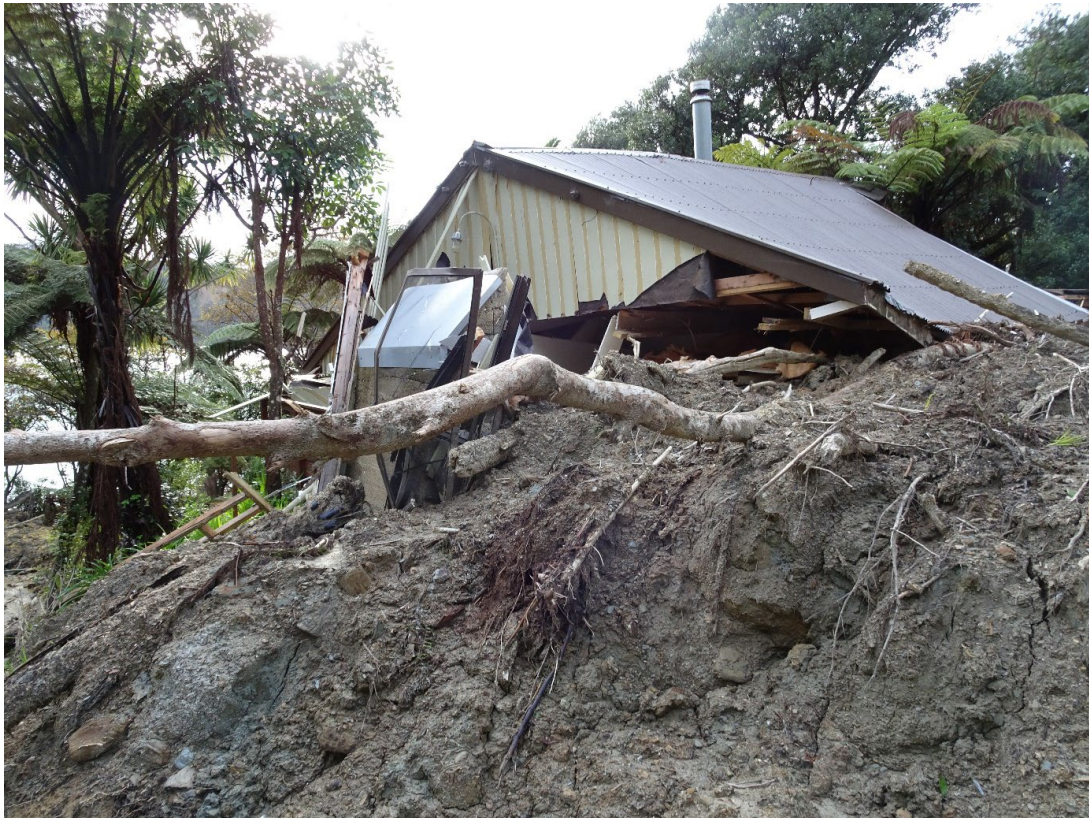
Figure 5.4 Damage to a building from large debris flow.
