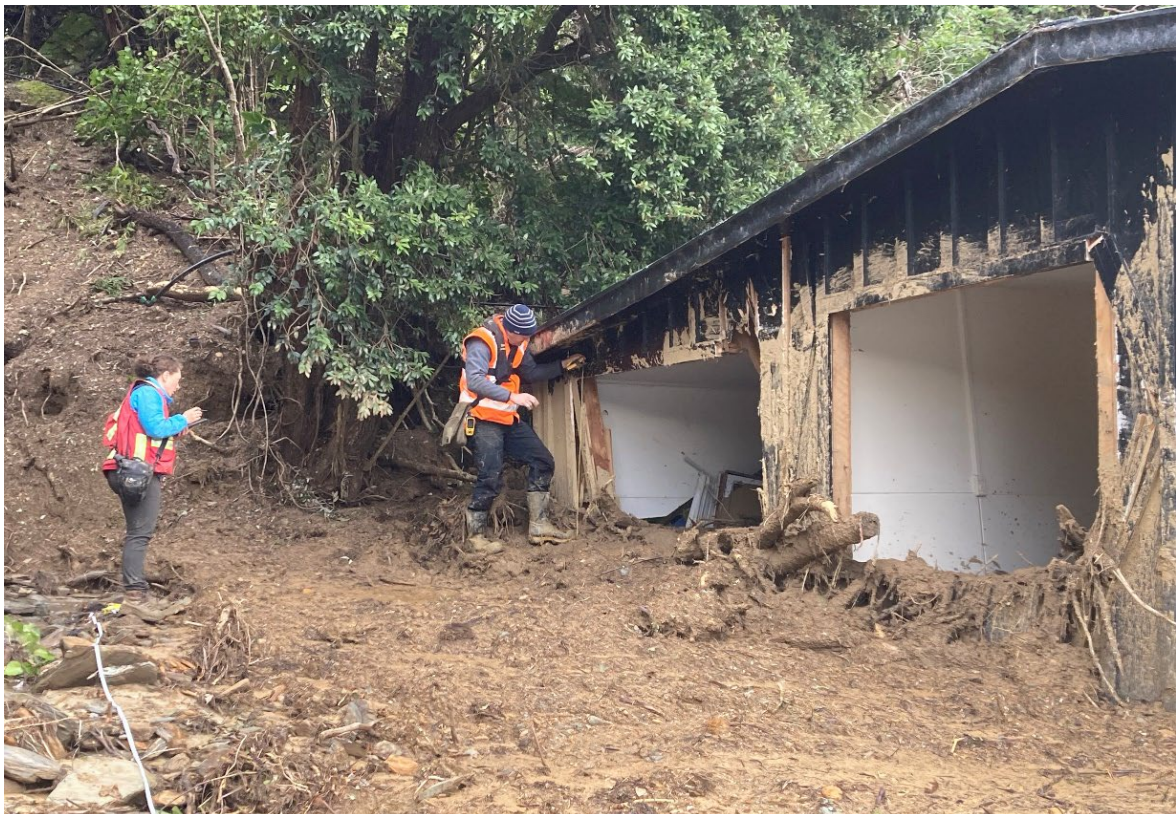
Figure A3.2 Surveying of landslide debris; measuring inundation along building side. We measured maximum run-up signs (here, above the building windows) not the height of the debris at the time of survey (here, at the base of the windows).
