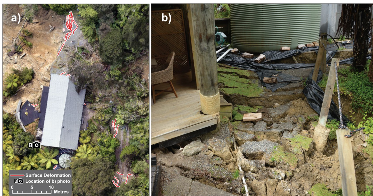
Figure 4.4 Example of surface deformation (cracking) at LS 22-3. (a) Location of cracks mapped from orthomosaic photos. (b) Extensive cracking obscured from the orthomosaic by vegetation.
