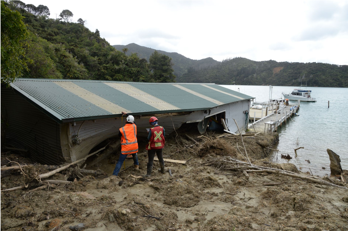
Figure 4.5 Inspecting and assessing structural damage to a boatshed impacted by a debris flow.
