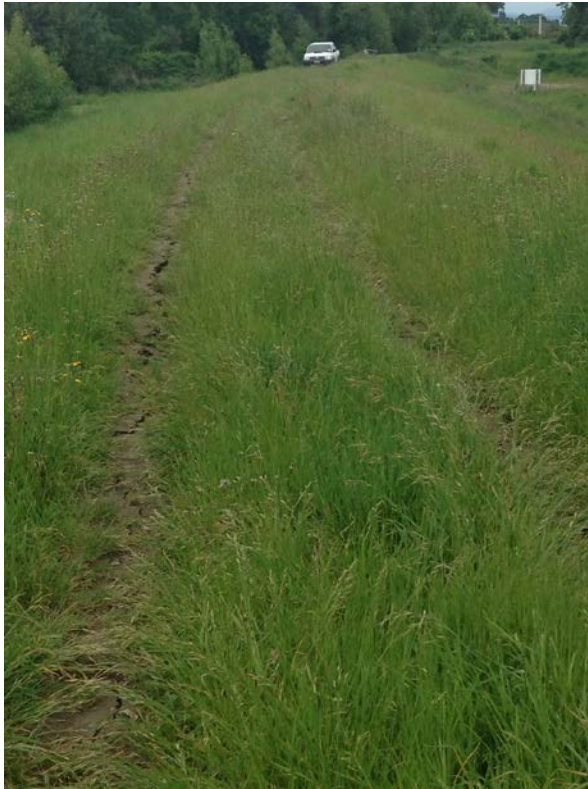
Figure 1 - Surface cracking of LW06 caused by lateral spread from the 2016 Kaikōura earthquake
