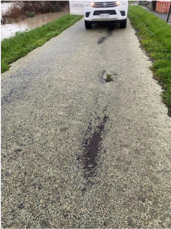
Figure 5 - Surface cracking of LW05 observed during July 2021 flood event, indicating internal failure
