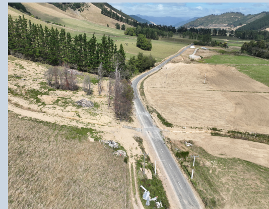
📷 Recovery repair works at the Ronga Road slip site are now complete
