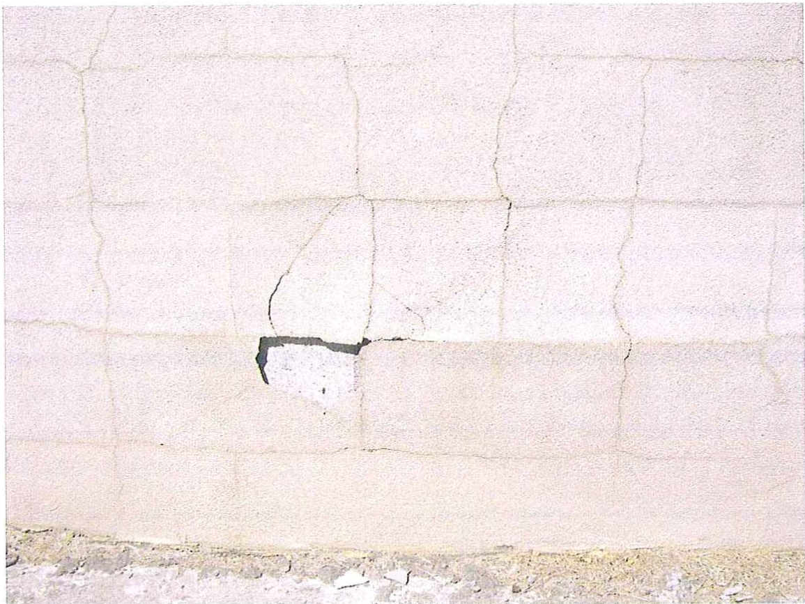
Plaster Cracking and Falling off Pine Hill Rise Sign
