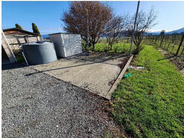
P7: Concrete pad located to east of garage, understood to be used for filling spray equipment.
