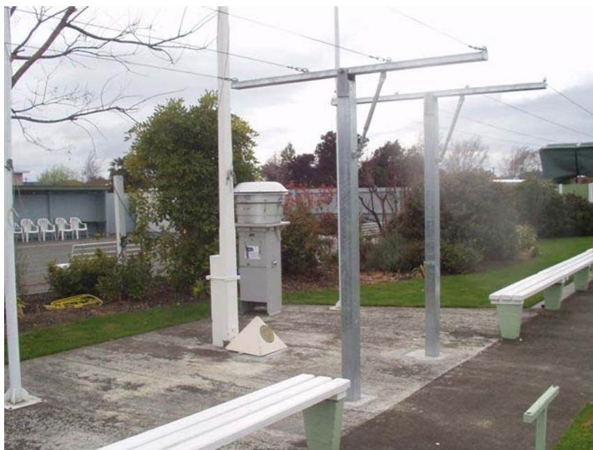
Figure 2.5: PM 10 monitor at the Redwoodtown air quality monitoring site
