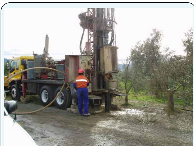
Figure 6.7: Top rotary drive rig. The top head drive is the square shaped object opposite the driller. Drill cuttings emerge from the round hole below this and have formed the wet patch on the ground. Two portable air compressors are required to drive the drilling process and provide air through the large hoses connected to the rig.
