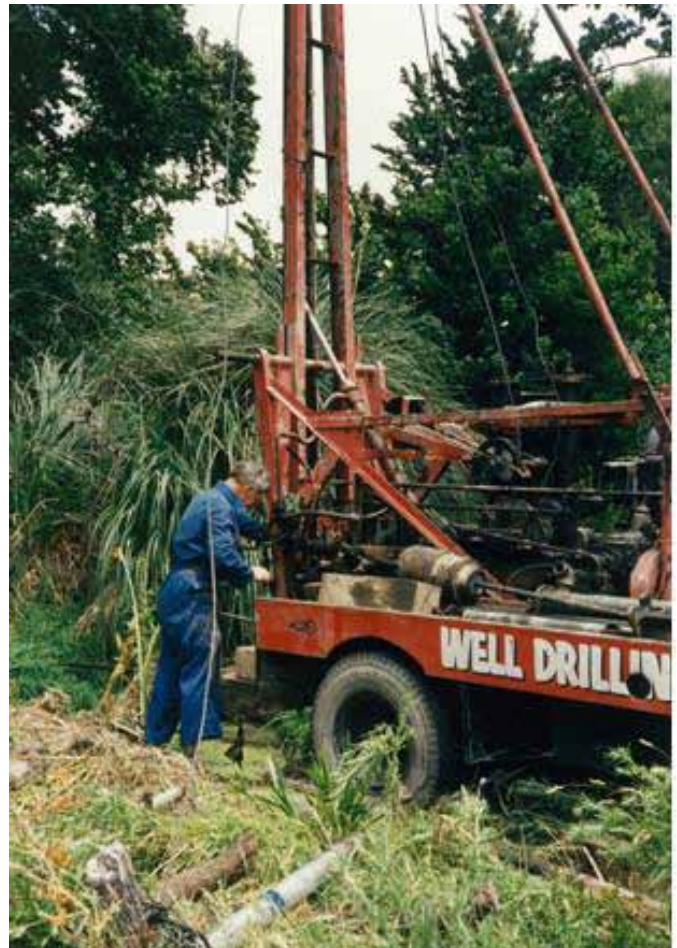
Figure 6.14: Mr Bob Thoms grouting a well at Riverlands in the late 1980s.
