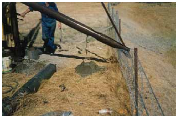
Figure 6.3: Sand pump in operation. Sand brought up from the well is falling from the hole in the bailer and gathering in a pile.
