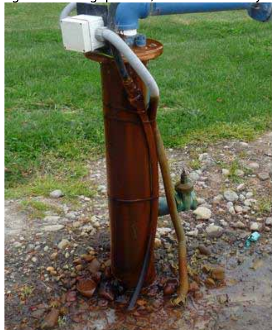
Figure 28.8: Staining on Fairhall Golf Club well headworks
