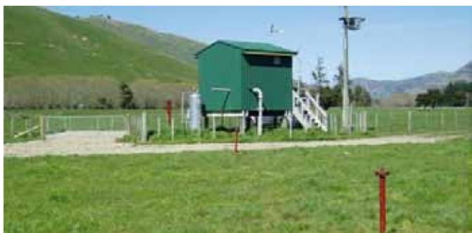
Figure 40.3: Havelock municipal supply wellfield
