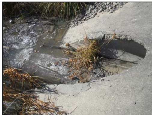
Winery wastewater in the stormwater system
