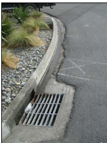
Wastewater in the stormwater system
