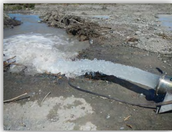
Figure 13: Uncontrolled discharge into the Awatere River
