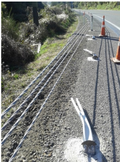
Damage to the newly installed wire rope barrier – Elevation, SH1
