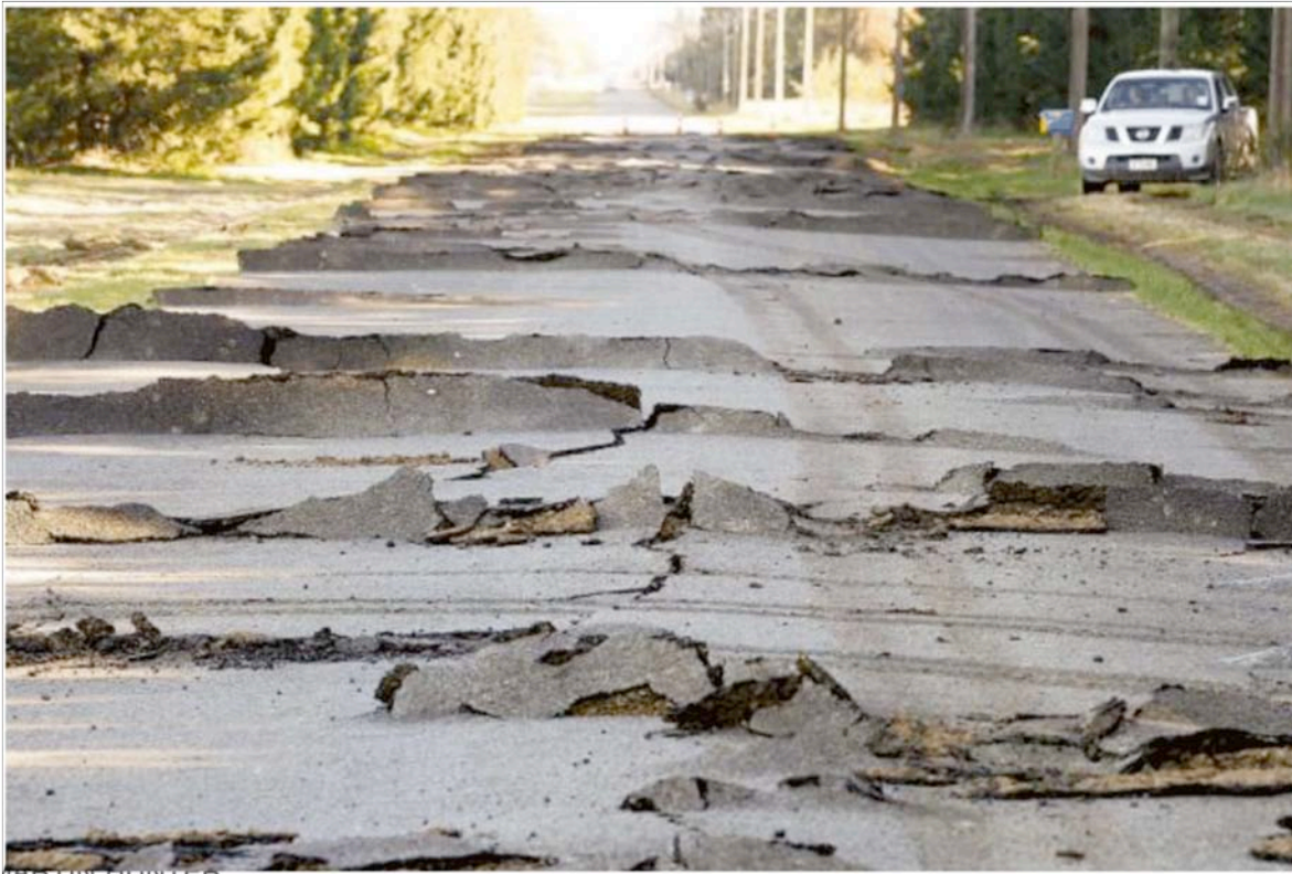
Figure 9. Fault Offset Through a Road
