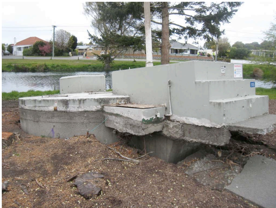
Figure 27. Floated and Tilted Wastewater Life Station 26, Porritt Park, Avonside
