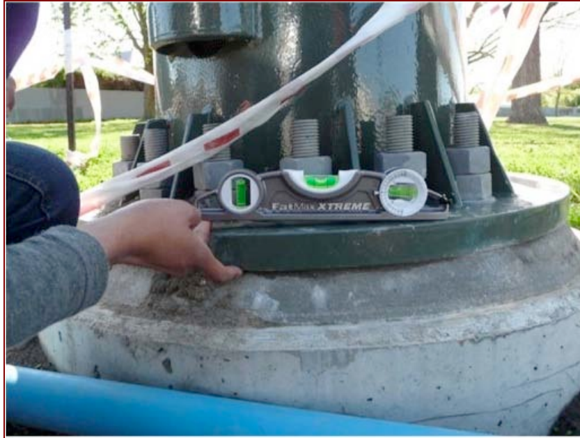
Figure 23. Cellular antenna tower out of plumb due to ground deformation.
