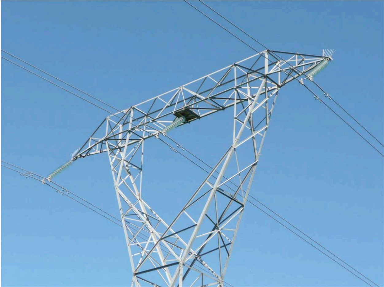
Figure 15. Displaced Insulators on Suspension Tower Adjacent to Fault Offset
