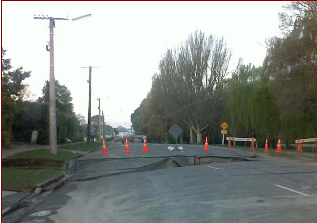
Figure 35. Road surface up heaving due to permanent ground deformation
