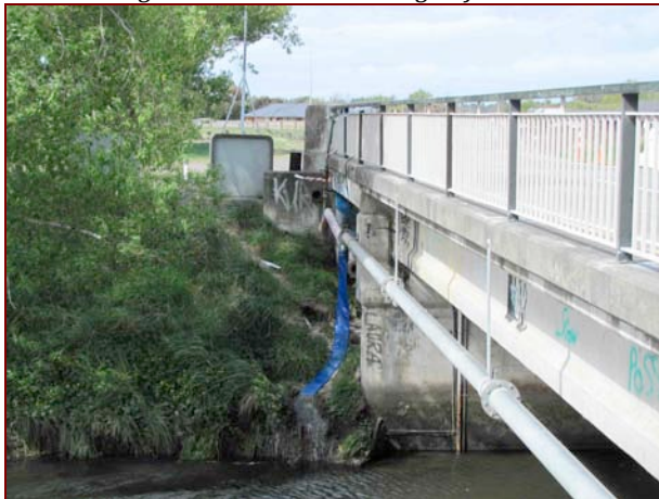
Figure 38. Plastic hose connected to broke pipe to discharge wastewater to stream
