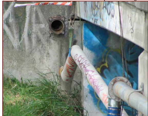
Figure 39. Close up of the damaged wastewater pipe
