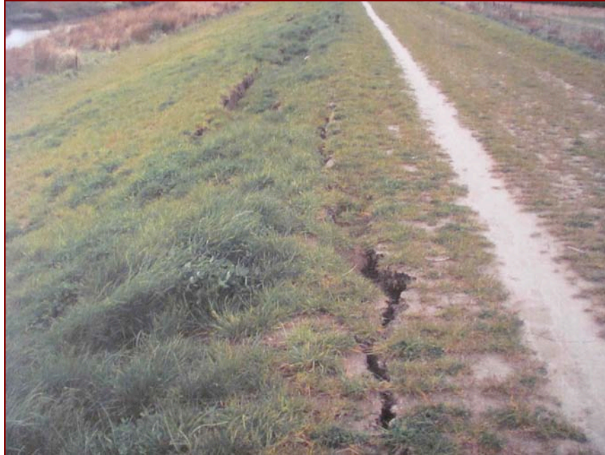
Figure 47. Moderate Damage - Stopbank
