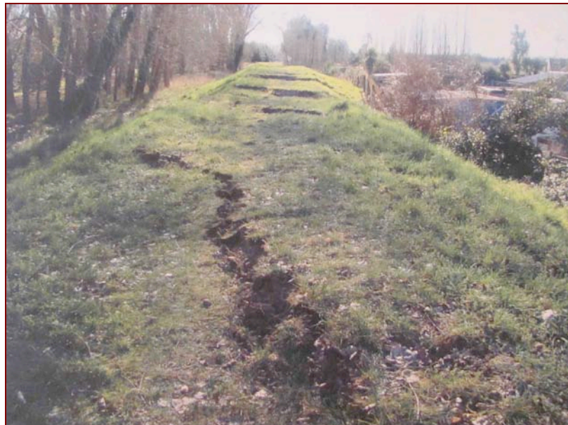
Figure 46. Major Damage – Stopbank
