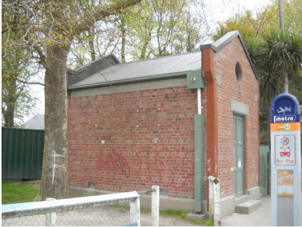
Figure 20. Orion URM Upgraded Small Substation
