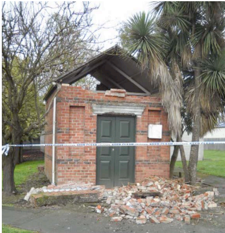
Figure 21. Orion URM Non-Upgraded Former Small Substation
