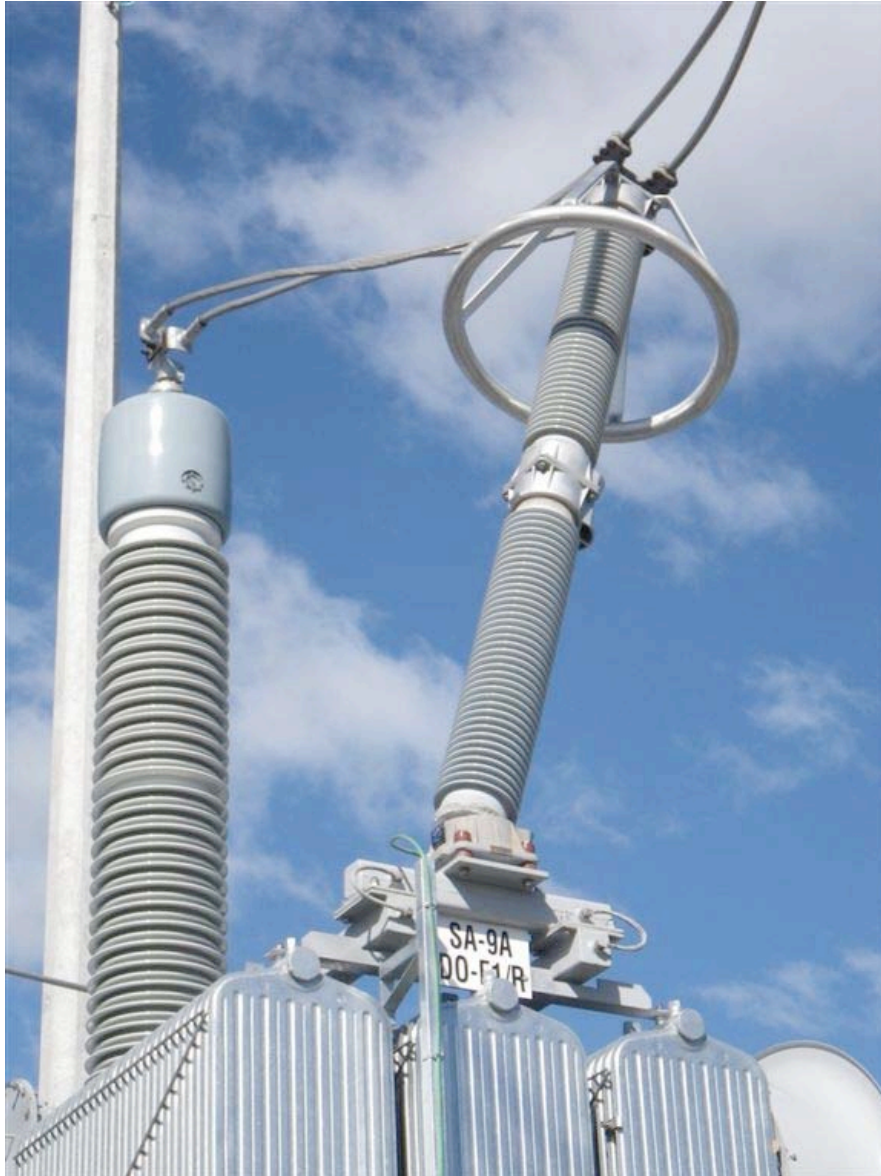
Figure 16. Broken Lightning Arrester
