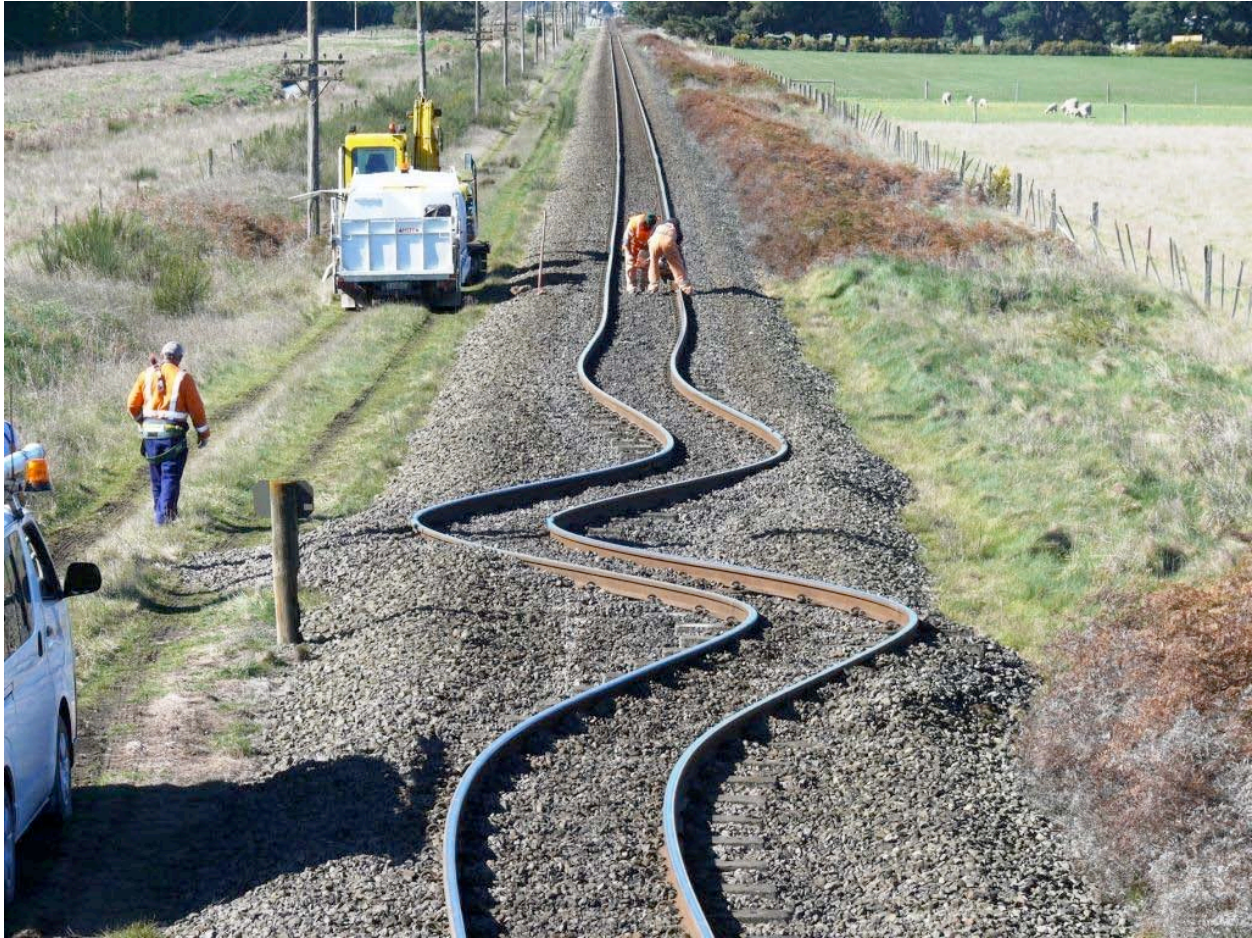
Figure 41. Buckling of Rails at Fault Offset Location
