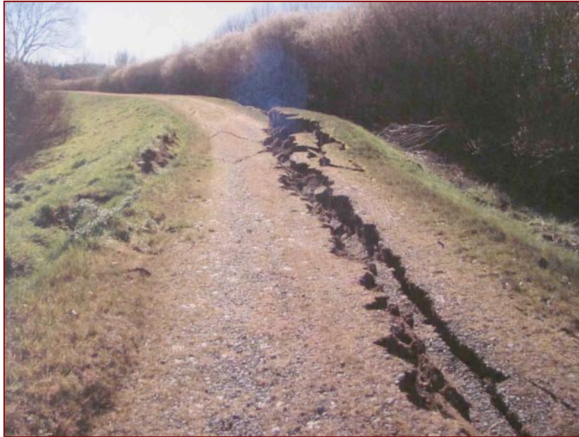
Figure 45. Severe Damage – Stopbank
