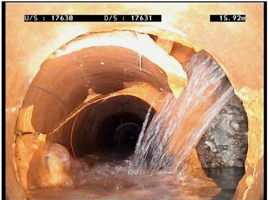
Figure 30. CCTV picture of Broken Sewer, MDC
