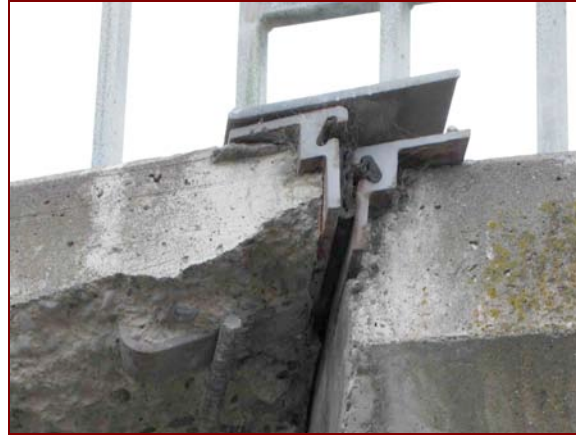
Figure 37. Deck and abutment impact damage
