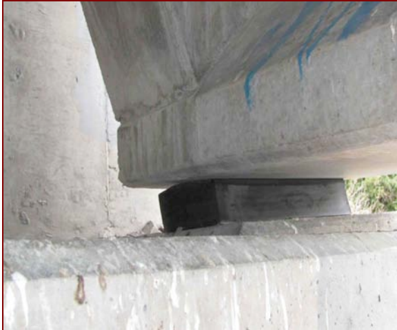
Figure 36. Rubber bearing deformed
