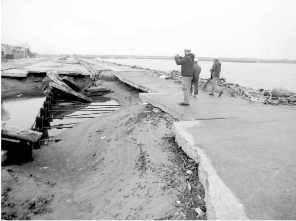
Figure 10. Significant scour behind the sheet pile-supported quay wall structures exposing the quay support sheet pile system in Otsu Fishing port, Ibaraki prefecture, Japan. Source (Chock et al. 2013)
