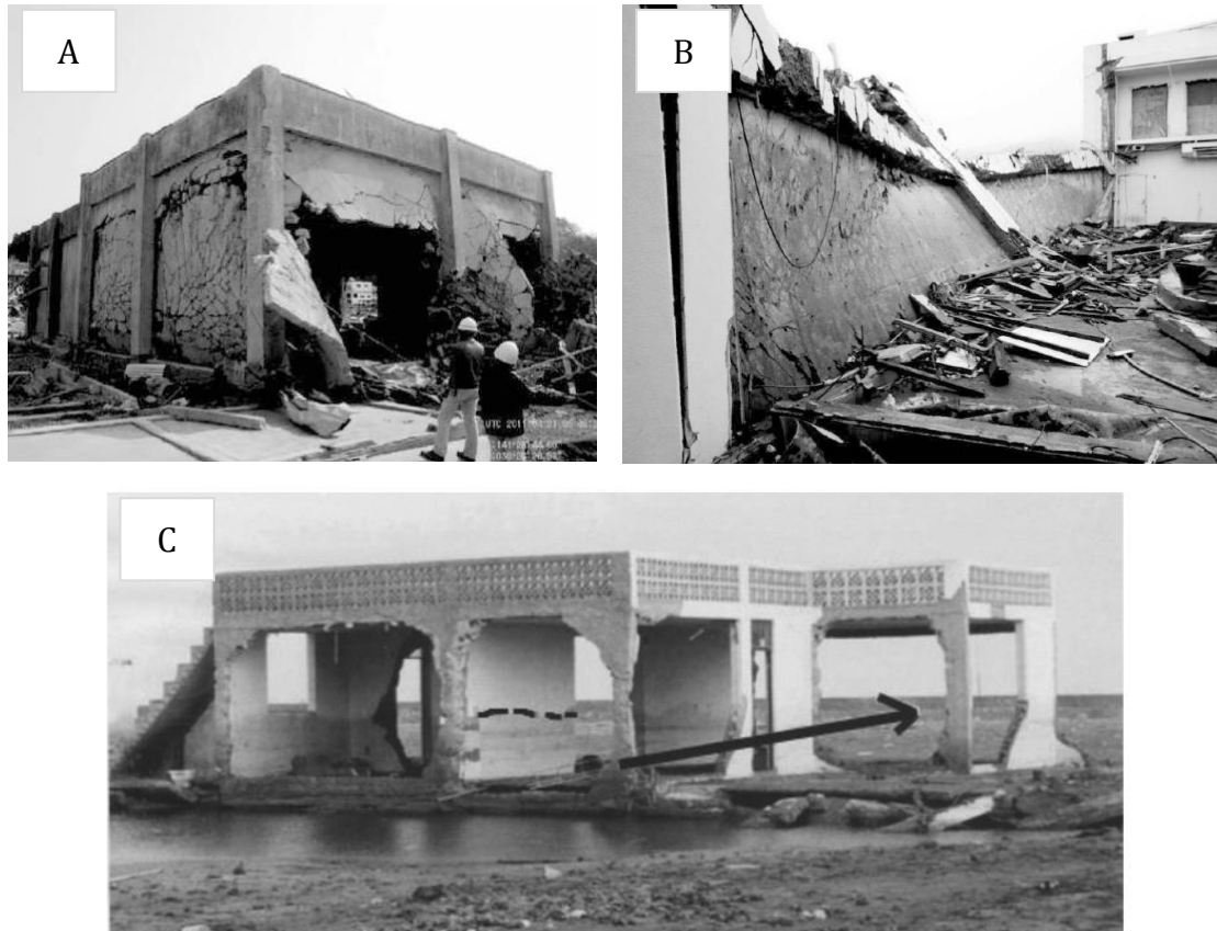
Figure 14. (A) Shear walls blown outward in a reinforced concrete building in Onagawa, Japan from the flow returning to the ocean during the 2011 Tohoku tsunami. Source (Chock et al. 2013). (B) Collapse of a steel framed multi-barrel vaulted roof due to the failure of load bearing walls (reinforced concrete pilasters and attached concrete shear walls infilled below the arch) from fluid lateral forces in Rikuzentakata, Japan. Source (Chock et al. 2013). (C) Damaged summer home in La Punta, Peru. Walls perpendicular to the direction of flow (black arrow) or parallel to the shoreline failed. Dashed lines show the stagnant water mark. Source (Okal et al. 2002)
