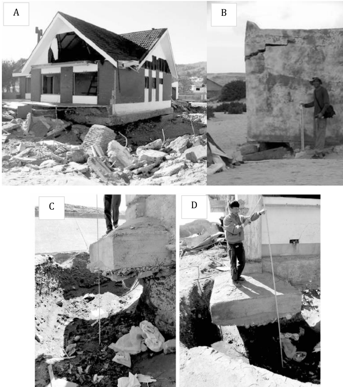
Figure 137. Examples of corner scour: (a) damage to a home in Dichato, Chile. Source (Edge et al. 2013). (b) Far-field effects from the 26 th December 2004 tsunami in Xaafun, Somalia showing scour damaged a house corner. Source (Fritz & Borerro 2006). (c-d) 1.4m deep scour pit below a buildings foundations behind a failed seawall in Tarou, Japan. Source (Chock et al. 2013).
