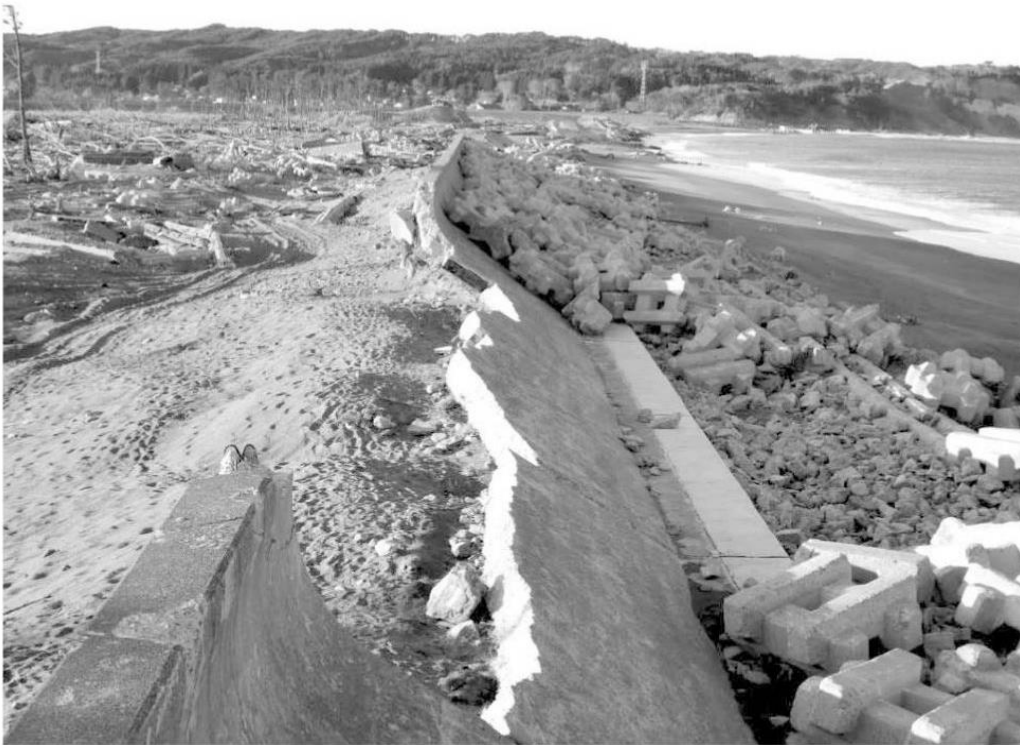
Figure 9. The front of a damaged earth filled and concrete lined seawall at Noda, Japan after the 2011 Tohoku tsunami. The seawall had a parapet lining the crest but failed in many locations due to the loss of internal earth fill from scouring. Failure also appeared to be concentrated at the junctions between adjoining segments of seawall, resulting in a large number of armour units being displaced inland. Source (Chock et al. 2013)
