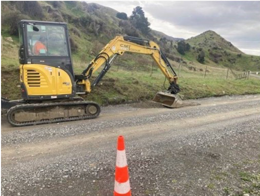
Surface and water table repairs at RP 980 - the Grey River Bridge, between Limestone Bridge and Moleswo
