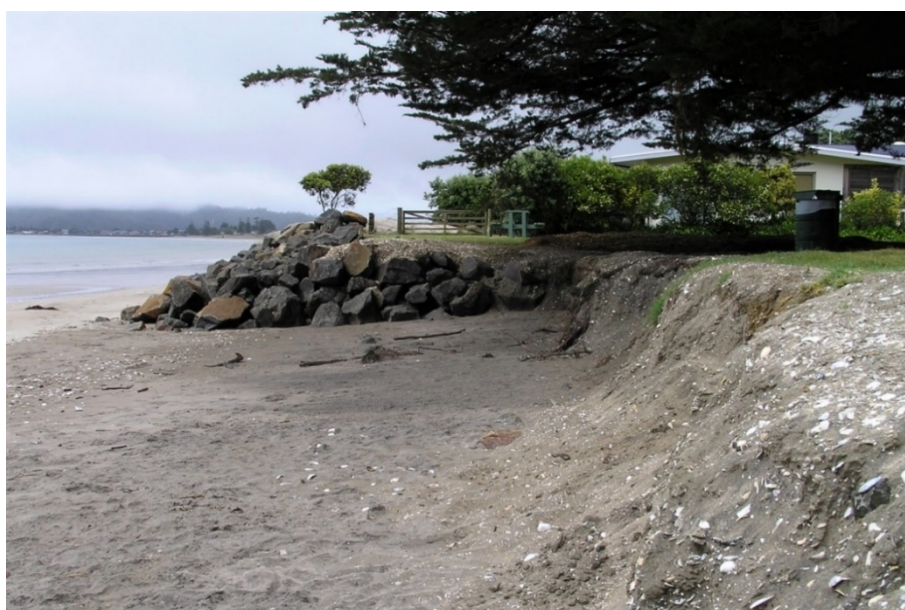
Figure 9-3: Erosion beside a sea wall in Whitianga. Photo: R. Bell, NIWA.
