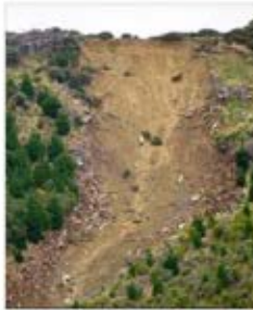
SMASHED APART: A failed skid site in the Marlborough Sounds after the big storm at Easter.
