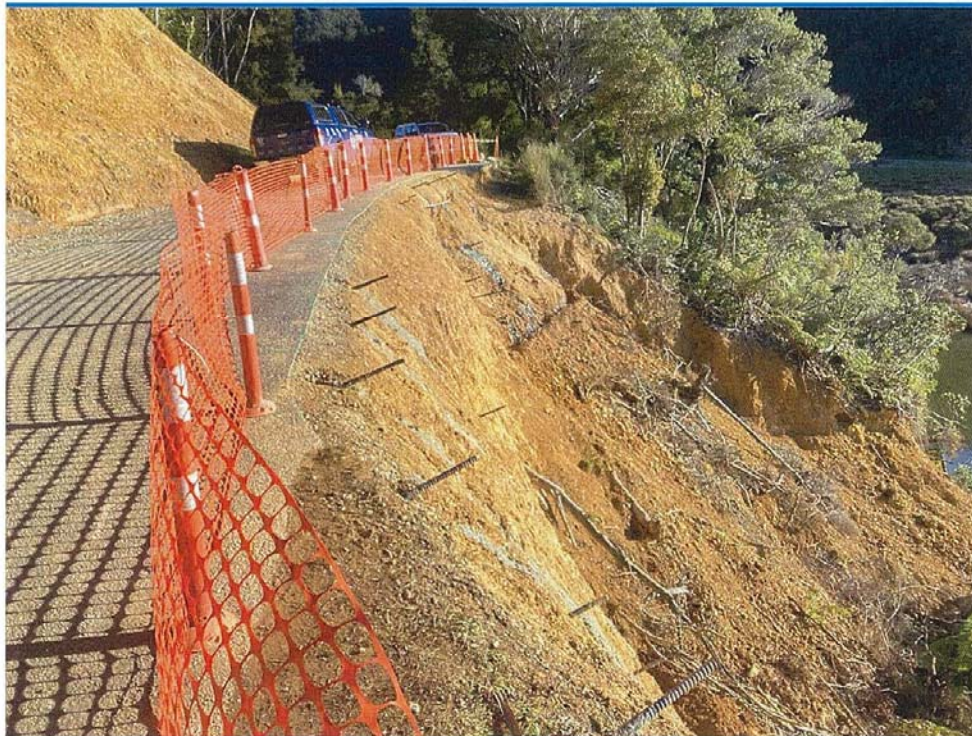
Nails have been grouted into the upper rows for the slope stabilisation wall
