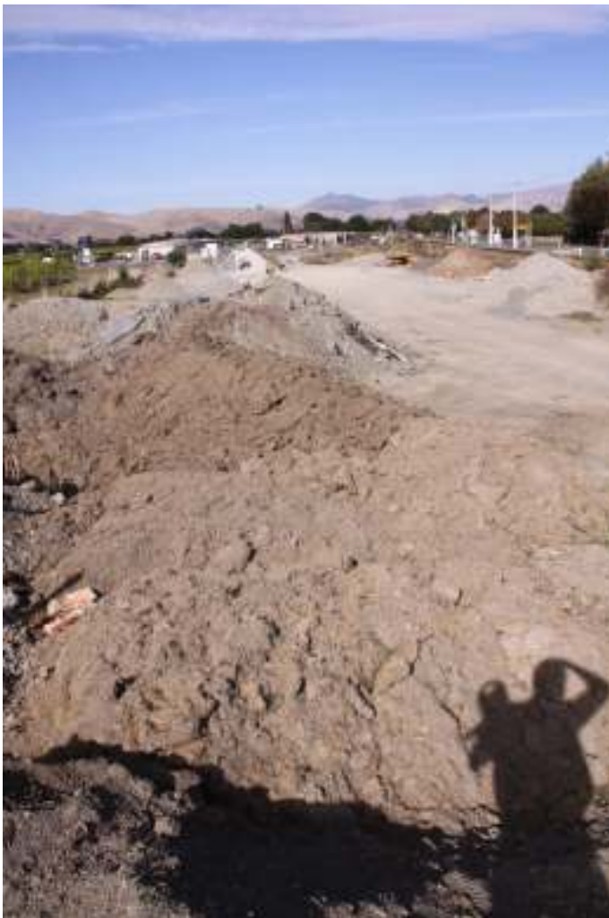
Photo 24: On-track. Powell Contracting. View of the site looking south from the middle of the site
