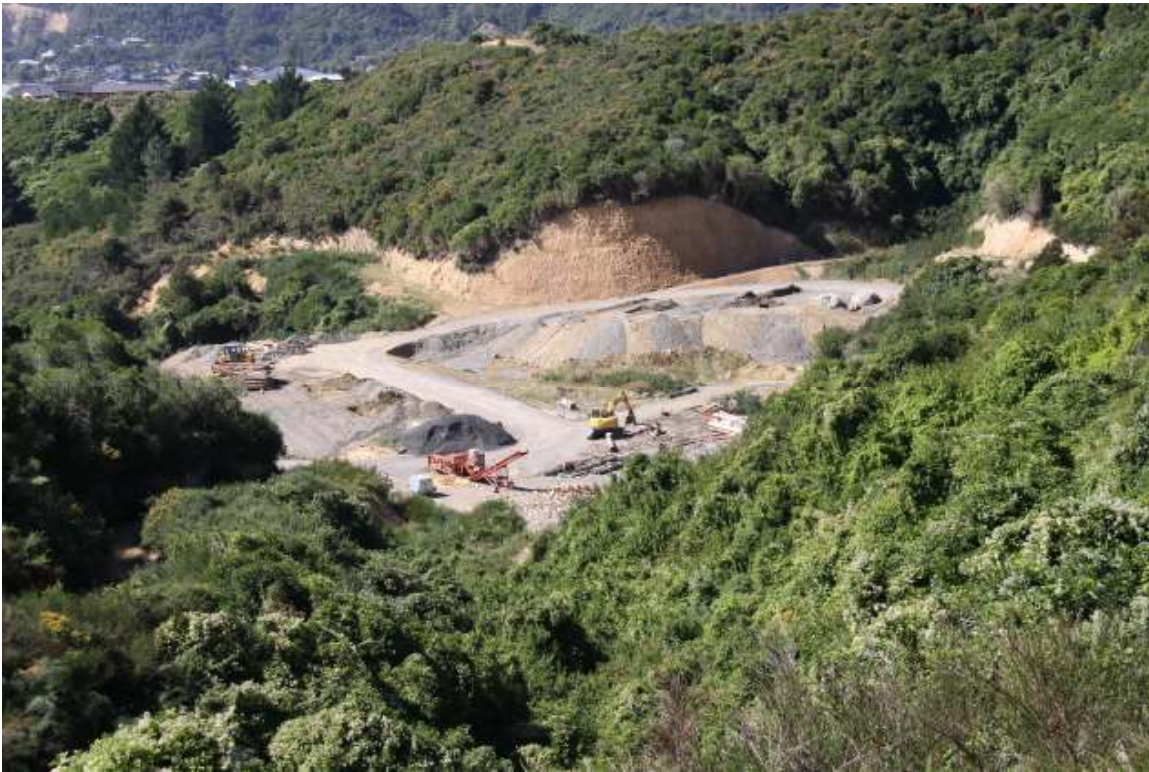
Photo 1: Picton Earthworks. View looking north east over the upper platform of the cleanfill site
