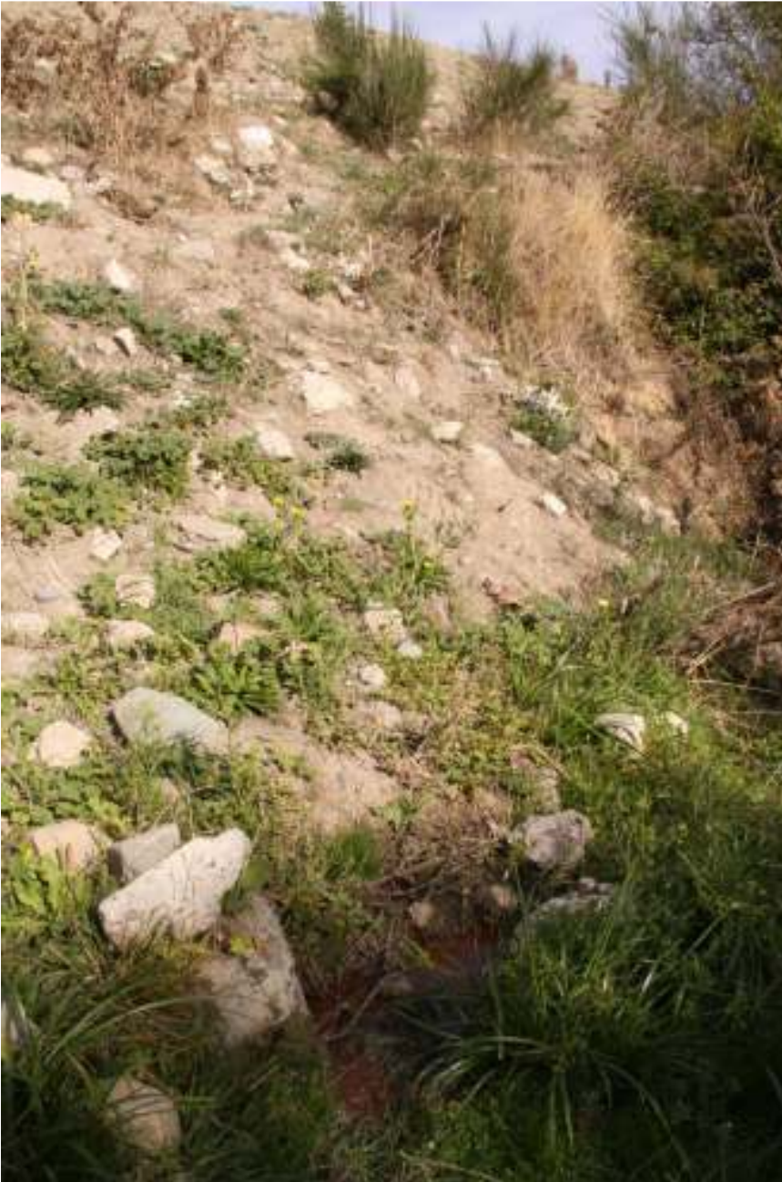
Photo 17: Taylor Pass Road - View showing leachate migrating from the base of the cleanfill site
