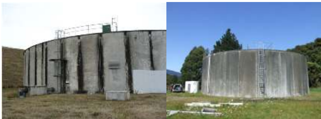
Figure 4-4 Pre-cast concrete slab and ferro-cement reservoirs at Weld Street Blenheim. The Elevation in Picton prior to seismic strengthening and upgrade.
