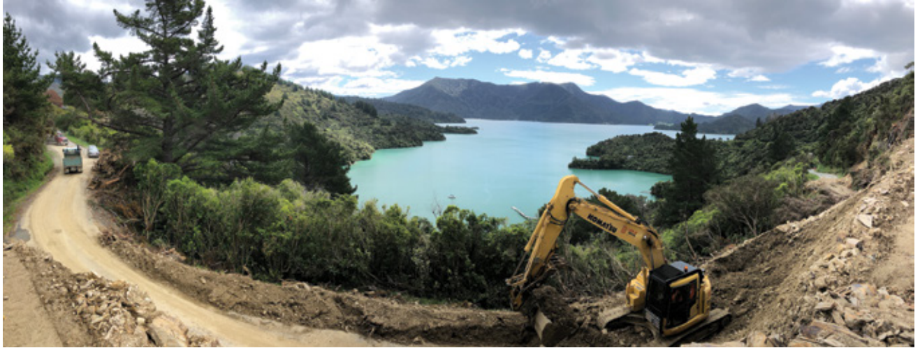
Damage to Kenepuru Road after the July 2021 storm.
