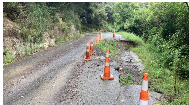
Figure 1-2: Underslip on Moetapu Bay Road
