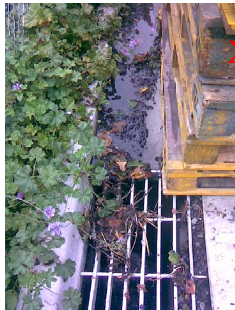
Grapes and Washwater entering Stormwater Sump
