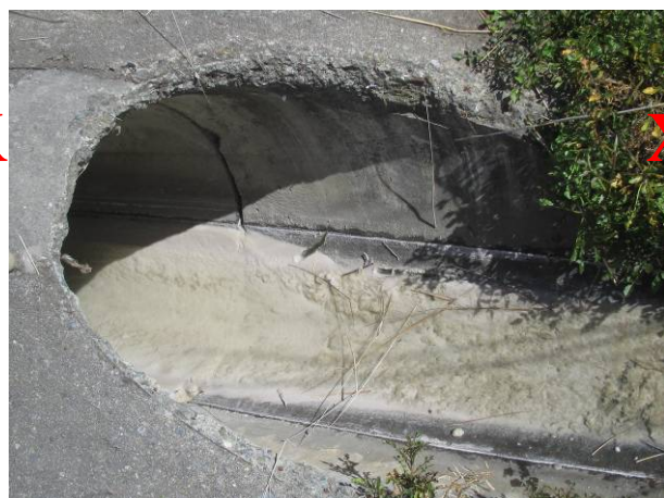
Stormwater Discharge Pipe Containing RDV Waste
