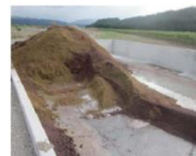
Sealed storage area with leachate collection
