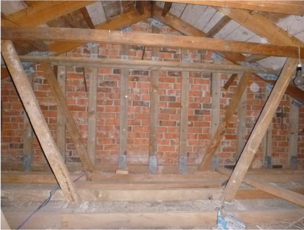
Photo 27: Brick gable wall with strong-back strengthening
