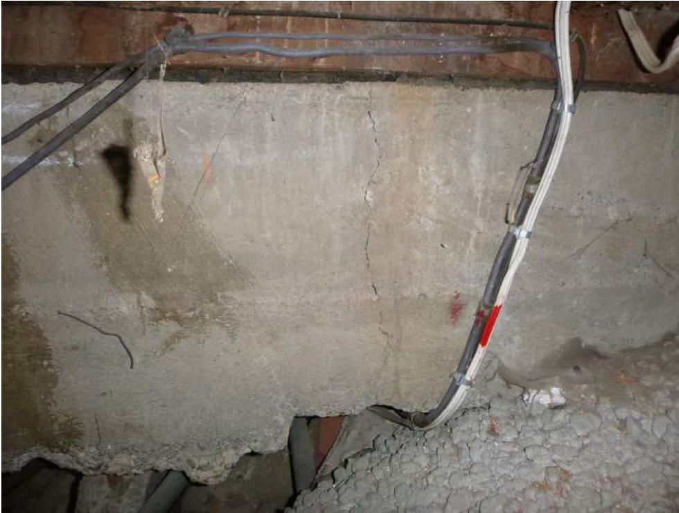
Photo 25: Crack in foundation wall at dining room
