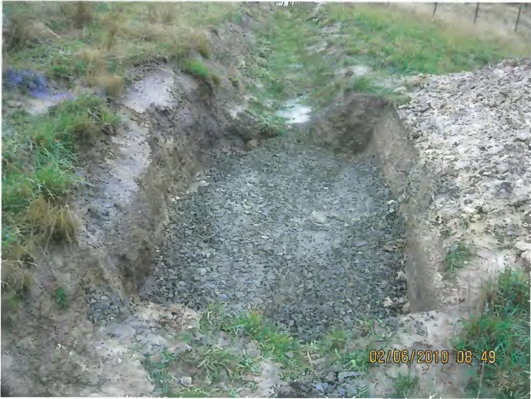
Under-runner being backfilled with road basecourse. This backfilling is limited to footprint of cut-off drain only.
