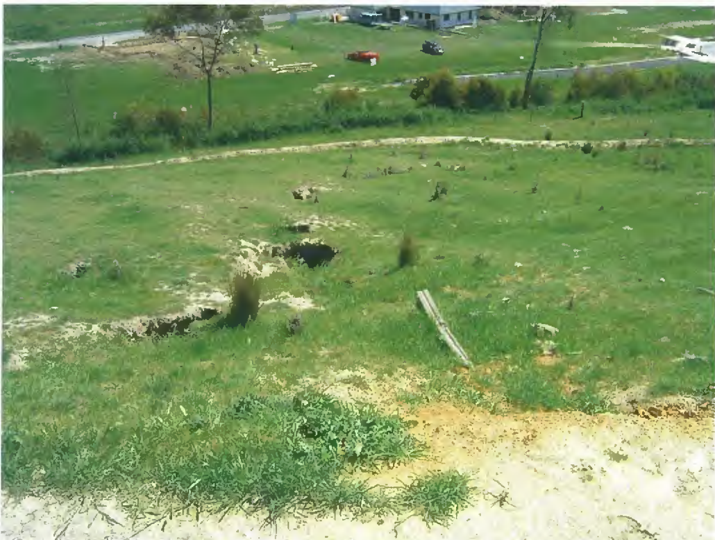
Looking down route of tunnel gully with cut-off drain running across background; shortly after initial construction in 2003
