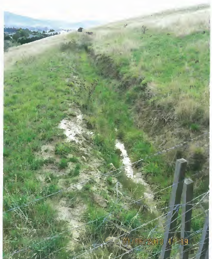
Cut-off drain in 2010. Grass growth in drain accentuating holding up water and ponding. Slumping of upstream bank of drain.
