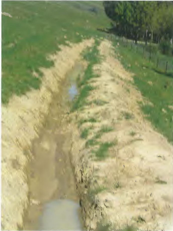
Cut-off drain at initial 2003 construction. Very flat grade of design has left ponding in drain with potential to seep down into tunnel gullies beneath.
