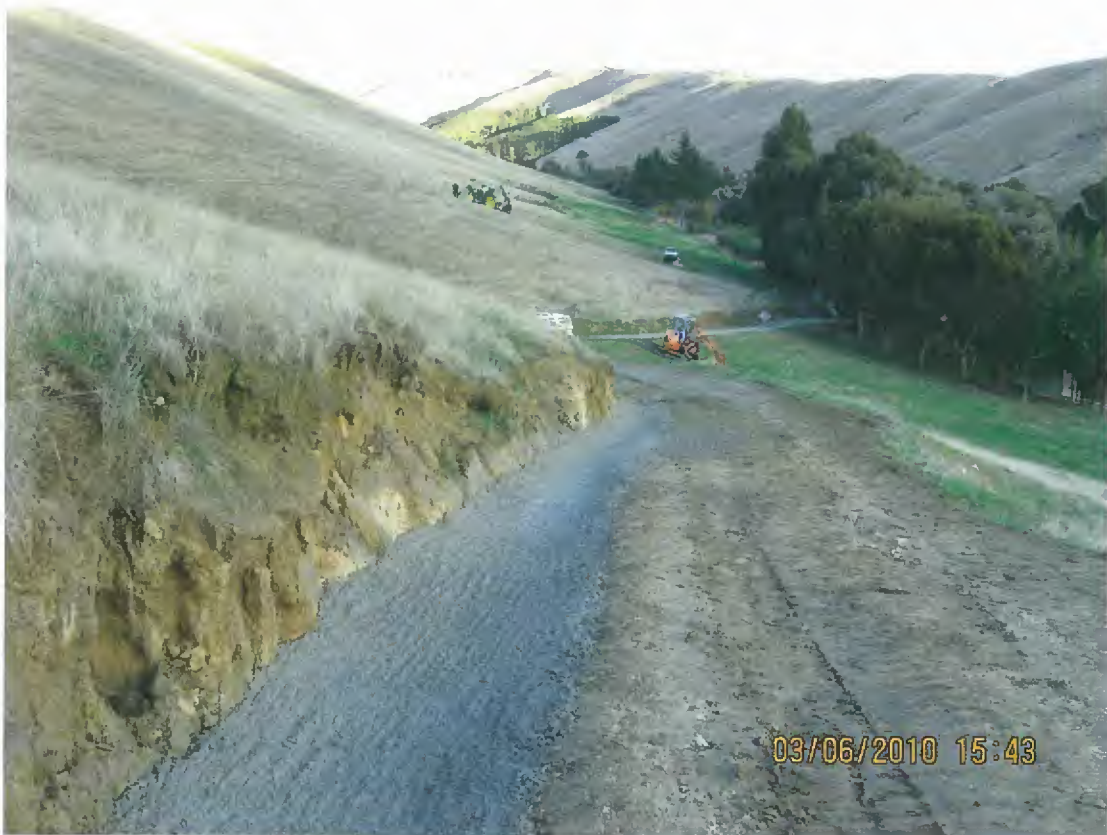
Farm access track tidied and backfilled with roading basecourse ("dirty AP65") and concrete slurry finish
