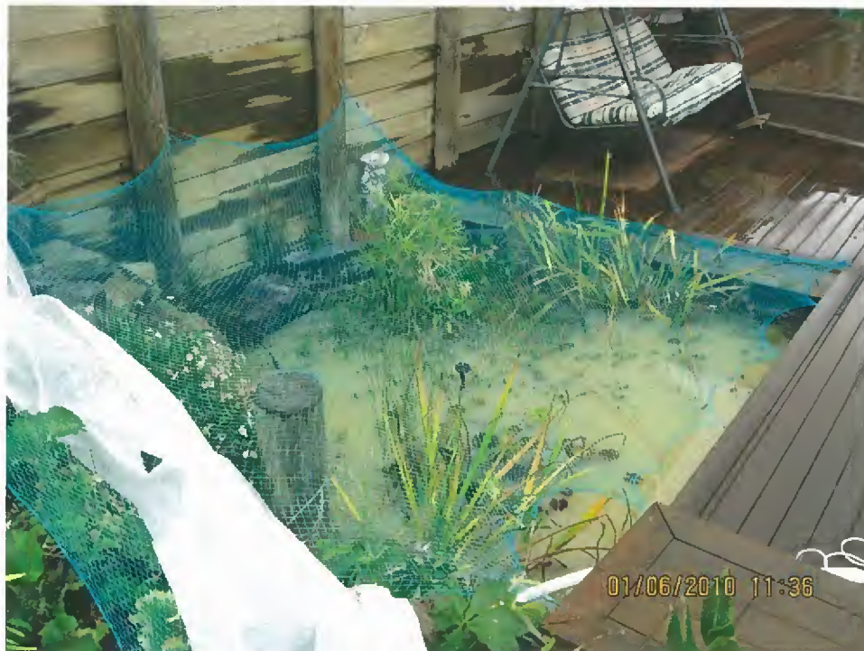
Dirty water ponding under Reed's deck
