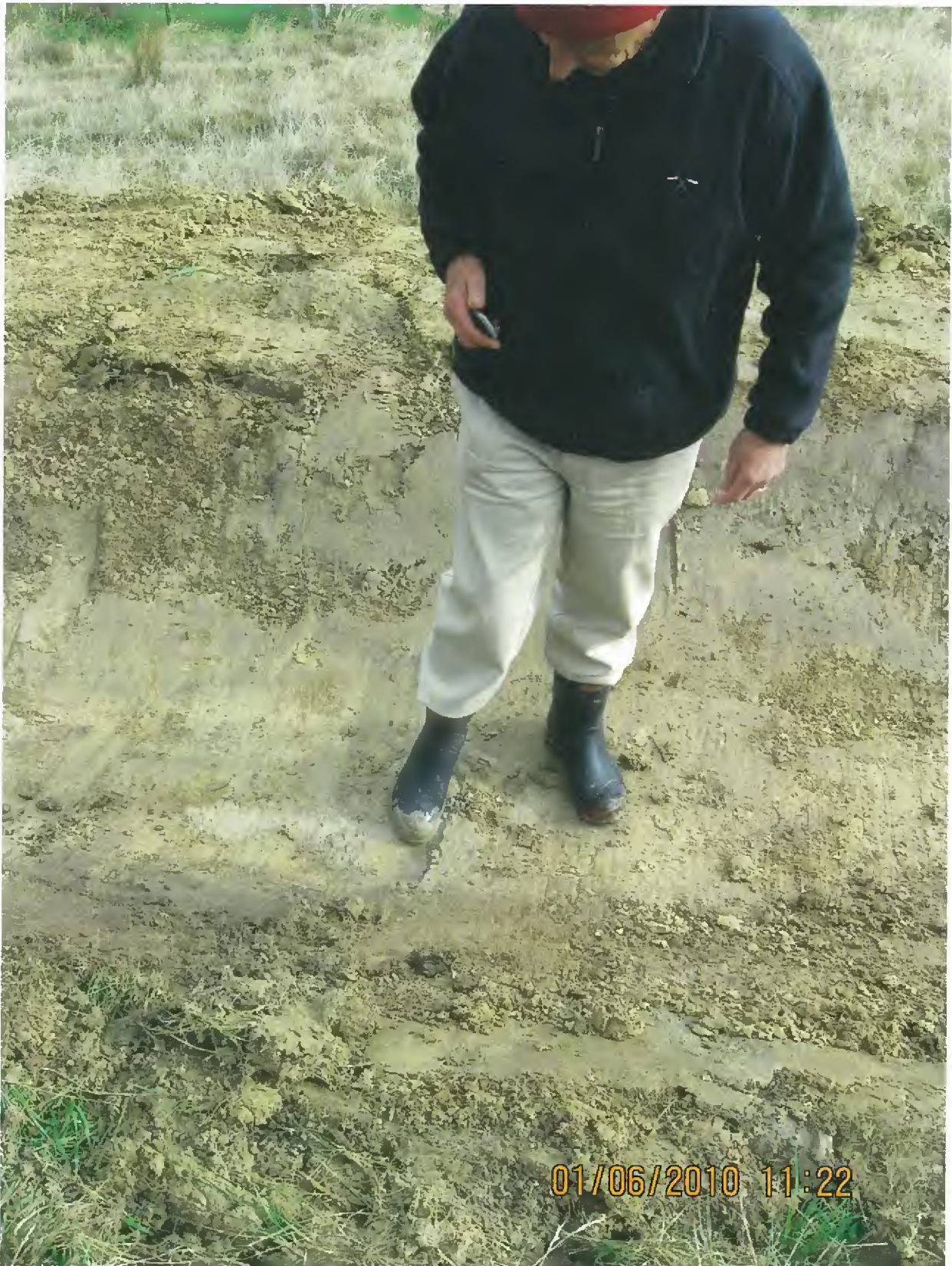
Seepage coming up through base of cut-off drain indicating incipient under-runner
