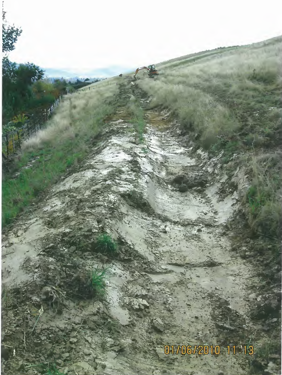
Cleaning out soil that has come down tunnel gully and filled cut-off drain
