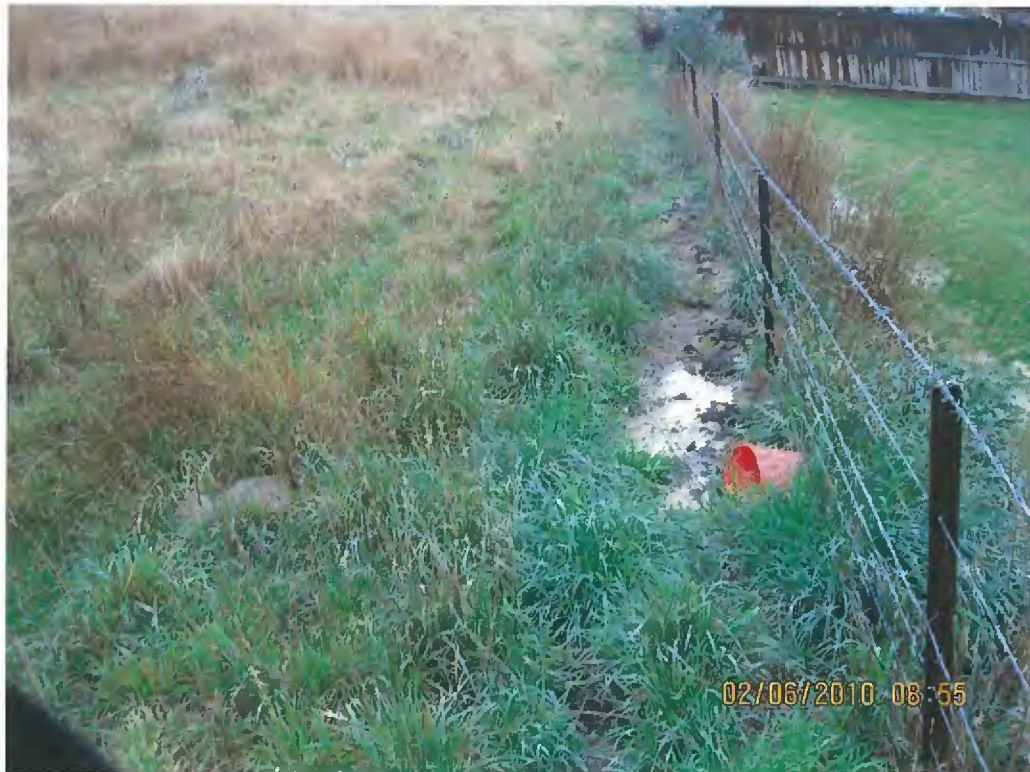
Possible potential problem to adjacent neighbour
