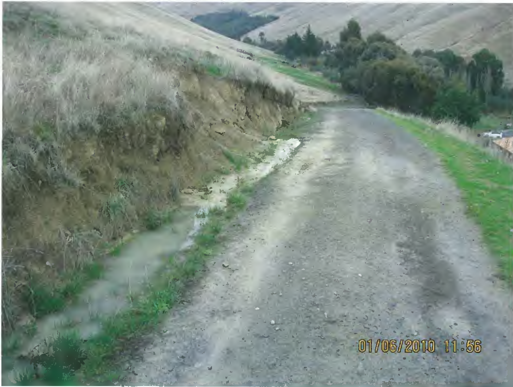
Farm access track higher up hillside. Water running along watertable before disappearing down hole into under-runner
