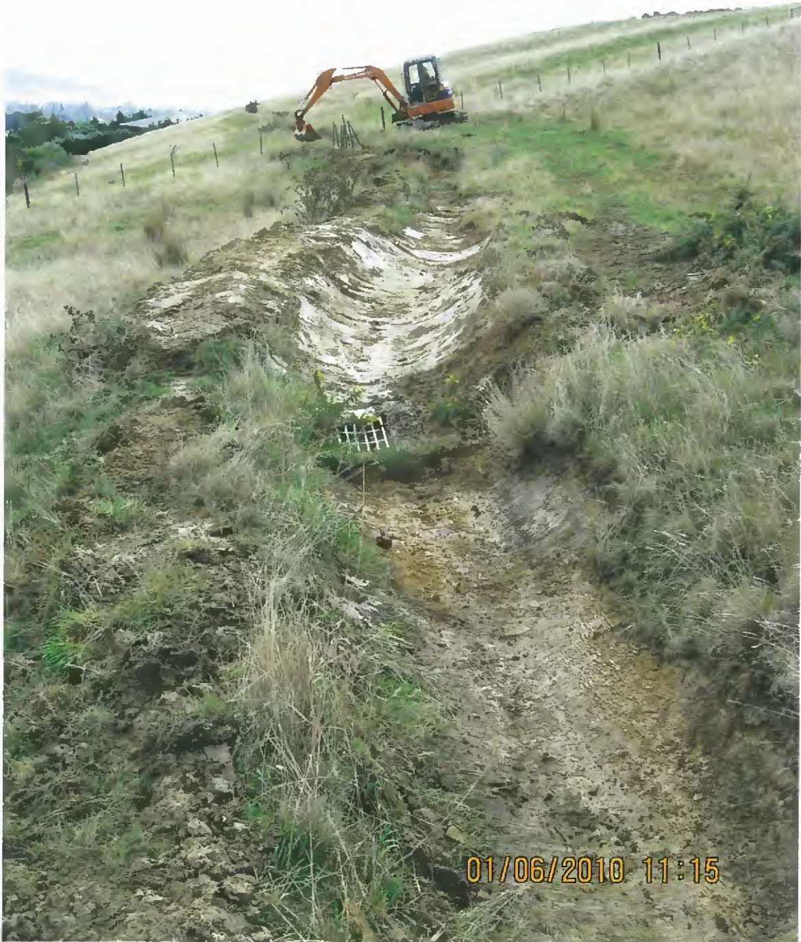
Cleaning out of drain has left sump higher than drain invert level; ponding must occur. Not reasonable to expect digger drive to excavate more delicately.
