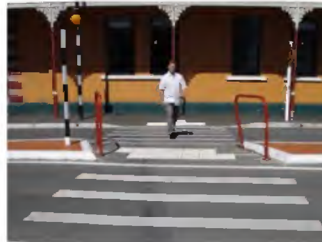
ABOVE FIG. 5-18: The column on the end of the crossing (behind the gentleman on the photo) could pose a safety hazard for the elderly and the disabled
