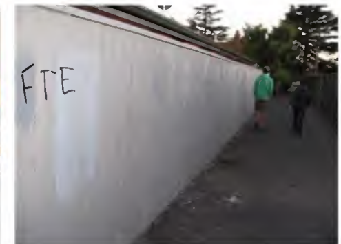
ABOVE FIG. 5-19: The signposted walkway between the CBD and Pollard Park has some safety issues
