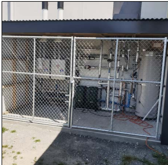
Fig 6 – Moutere Rugby Changing Rooms, new hot water gas calfont system and lock-up
