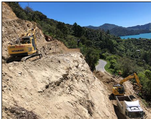
Approximately 2000m 3 of slip material has been removed this week from the Rock slip site
