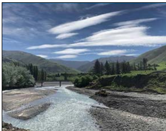
The river training on the Awatere River at the Limestone Bridge was completed on 6 November
