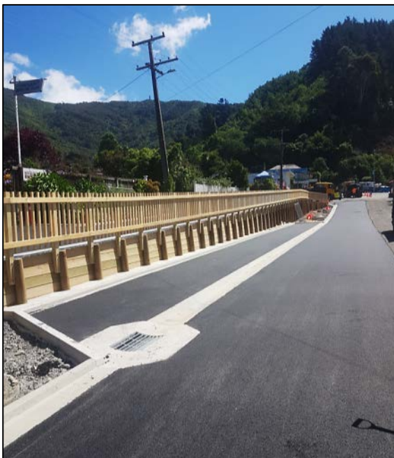
Fig 3 – Neil St Upgrade, new lower retaining wall and on street parking. Dec 2021
