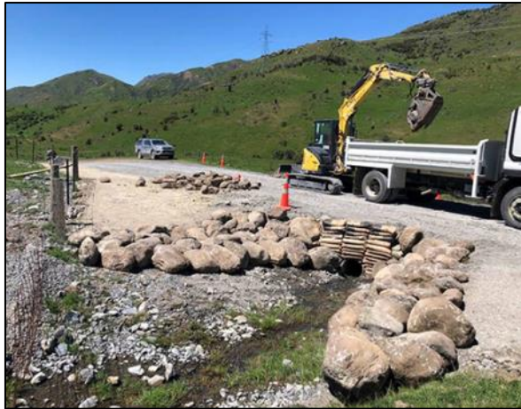
Road surface, water table and culvert improvement works 3.5km from the Limestone Bridge
