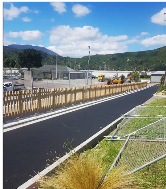
Fig 4 – Neil St Upgrade, sealed road and new retaining wall for residential and Havelock Bowling Green access
