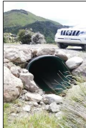
PE culvert with poor cover
