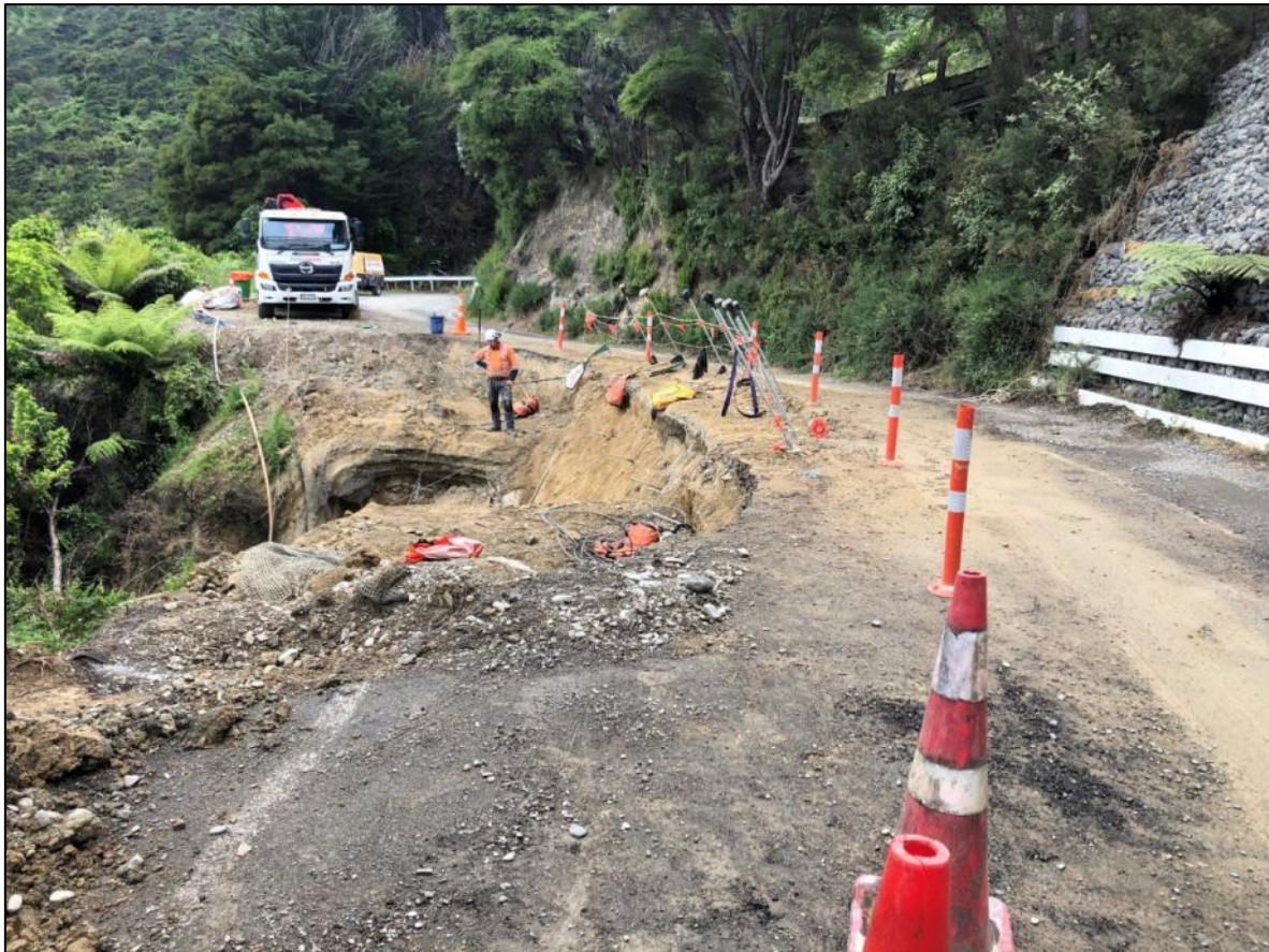
Figure 2-Slip stabilising at Portage
