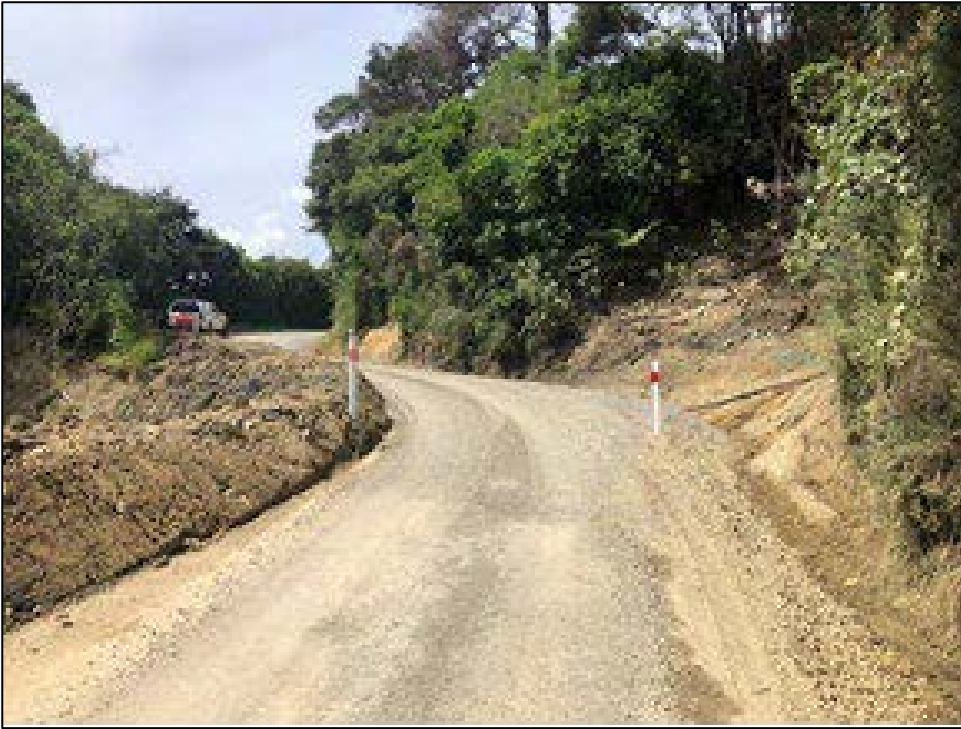
After improved access works have been completed on Kenepuru Road, just before Portage.
