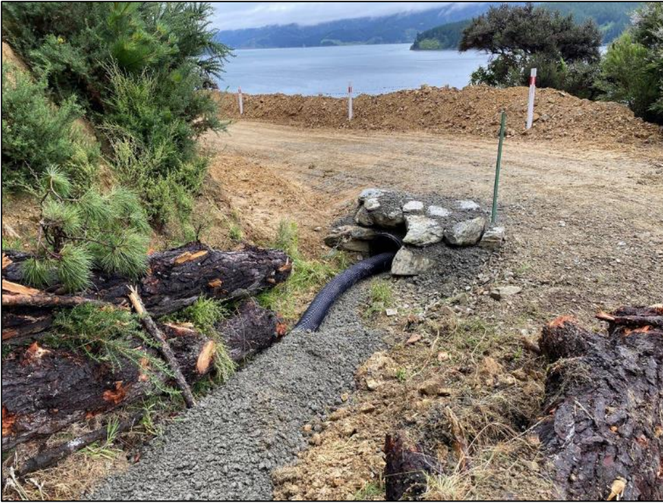
Temporary culvert installed to bypass storm water flow at 16.6 on Tumbledown Bay Road
