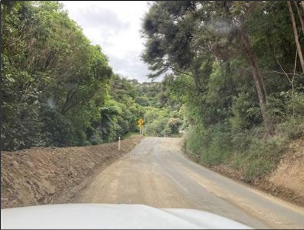
Improved access on Kenepuru Road, with earth bund installed to provide delineation and redirect storm water away from under slip.
