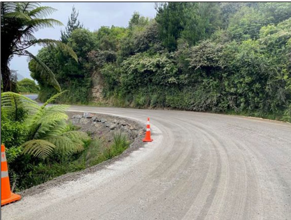
After works on Queen Charlotte Drive at Pukenui temporary shoulder rebuild for sealing.
