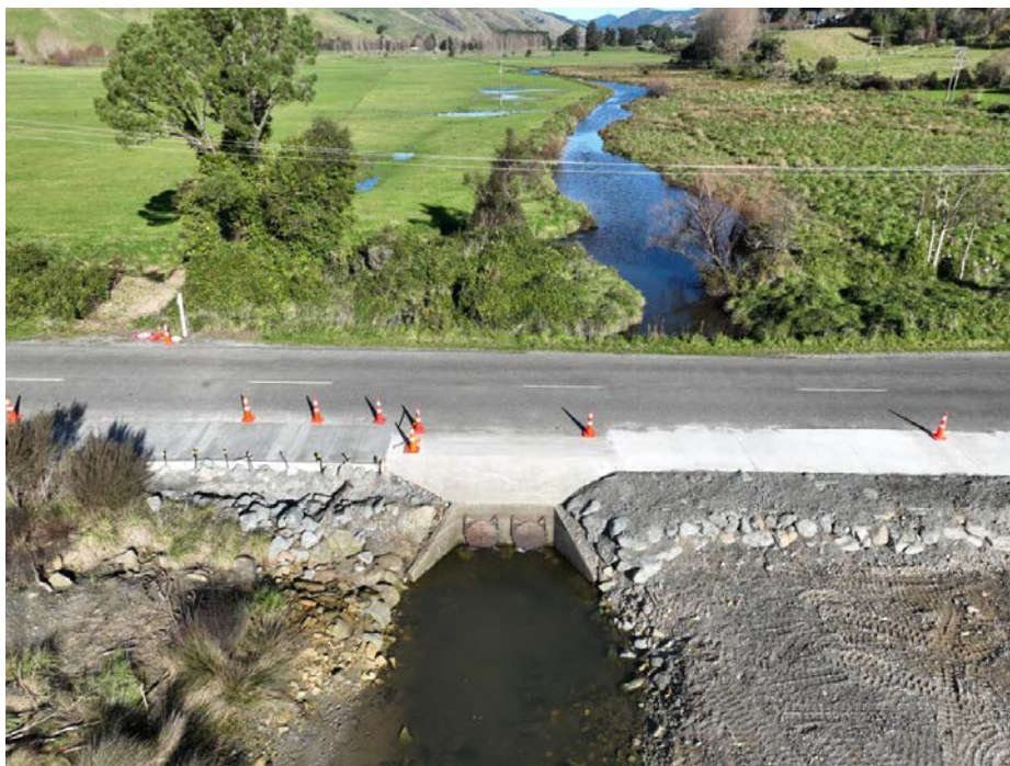
Scour repair completed on Queen Charlotte Drive causeway at Kaituna Estuary – image taken 31 May 2023
