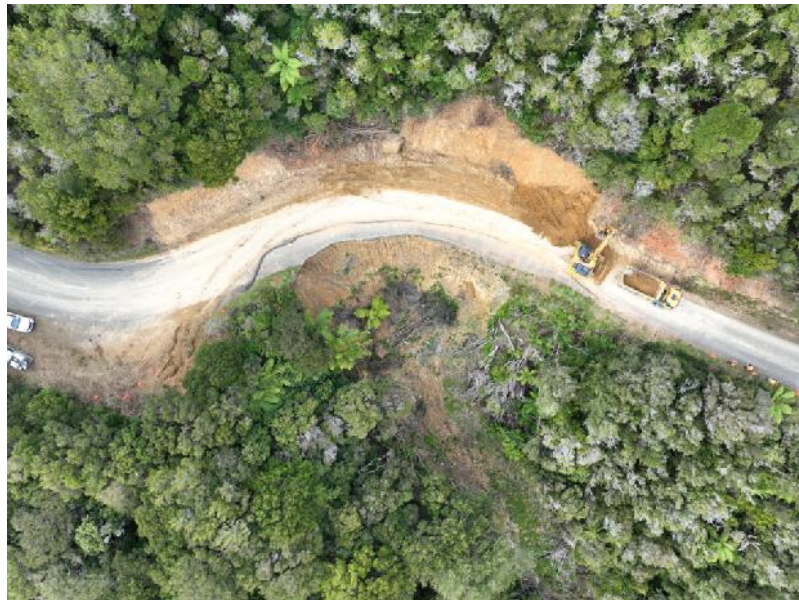
Repairs underway on Croisilles-French Pass Road at Fault FRP-518-11050 by Edridge Contracting
