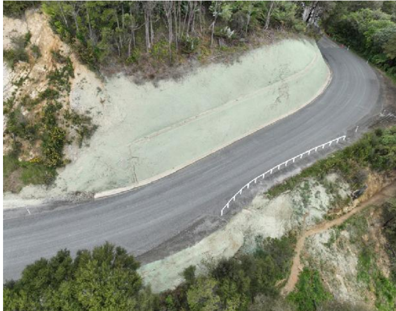
Hydroseeding on the completed retreat and drainage works on Queen Charlotte Drive Fault QCD-716-01156
