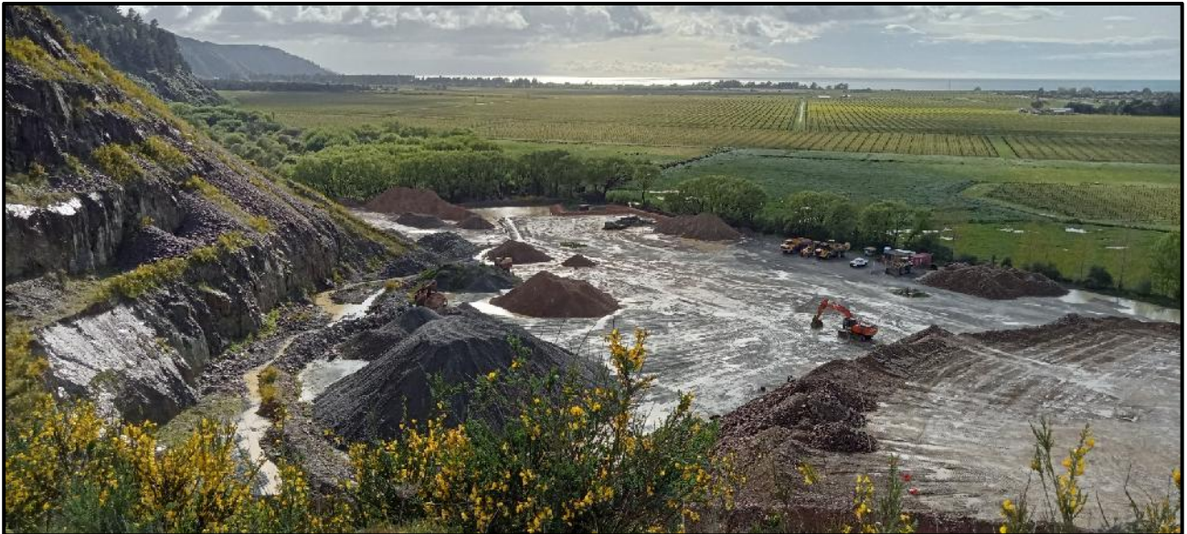
Figure 1 – very wet quarry floor, new settlement pond in the far corner
