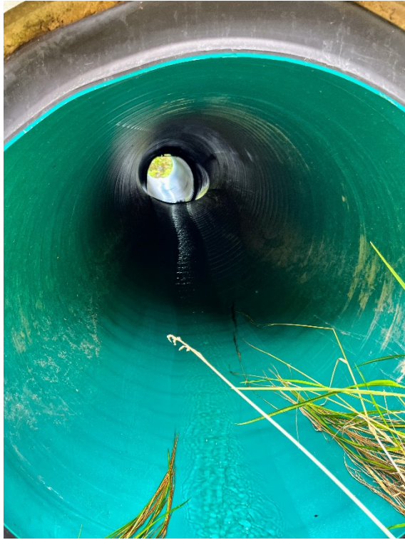
Fig. 15 – Deformed Culvert on the Main Road
