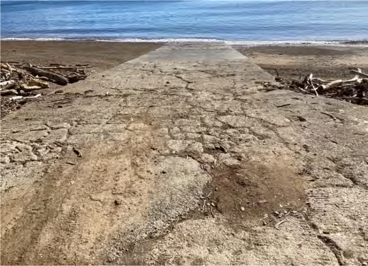
Concrete ramp in poor condition
