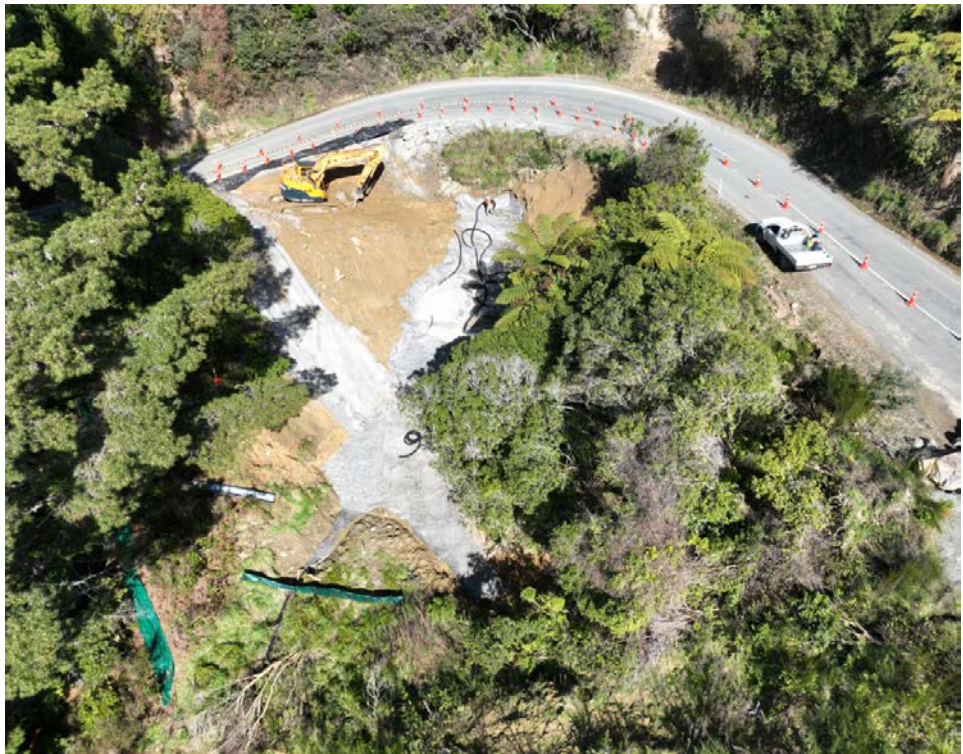
Repairs underway at Fault QCD-716-00514 with sediment fencing and a clean water diversion in place to manage erosion and sediment at the work site
