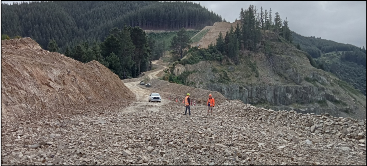
Figure 1 - West knob bench prepared for blasting, dumper traversing the upper quarry haul road in the background
