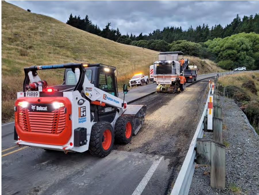
Figure 1 – Welds Pass Maintenance
