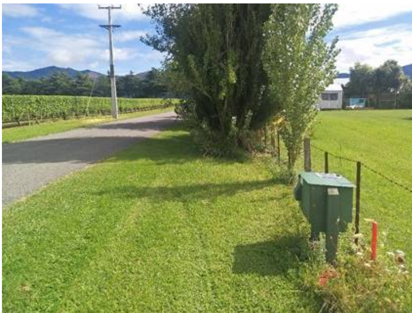
Photograph showing MDC Wratts Road monitoring well P28w3009. View looking north up Wratts Road towards Richmond Ranges with well on other side of green cabinet housing recorder instruments.
