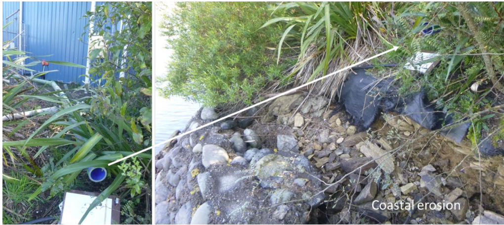
Figure 3. Observation of possible coastal erosion (exposed black geotextile mat and cavity at the top of the seawall) at outfall Site 26. However, the location of this outfall was not matched on Open Data / Smart Maps.
