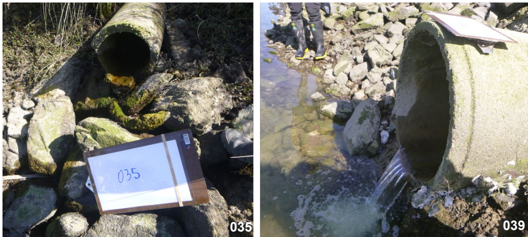
Figure 7. Outfalls (Sites 35 and 39) were observed to have baseflow during the site visit (dry weather conditions).
