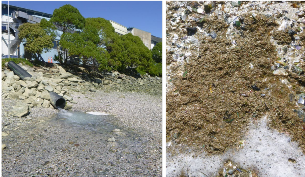
Figure 5. Observation of shell debris and mussel beard at outfall Site 24, possibly relating to consent U960064 (wastewater from a shellfish processing plant) and consent U110522 (which is added to the U960064 discharge stream).
