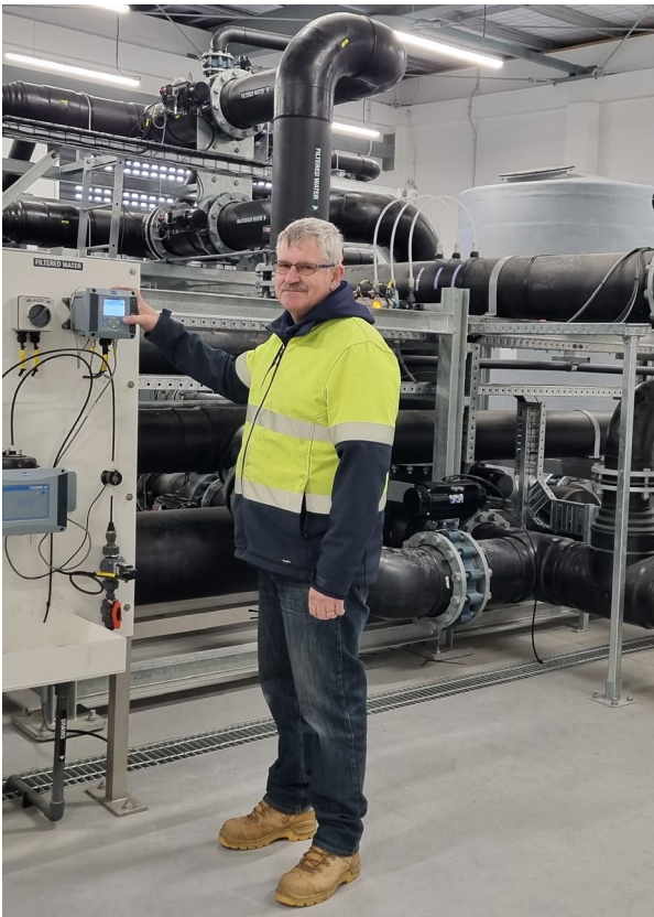
Renwick Water Treatment Plant
