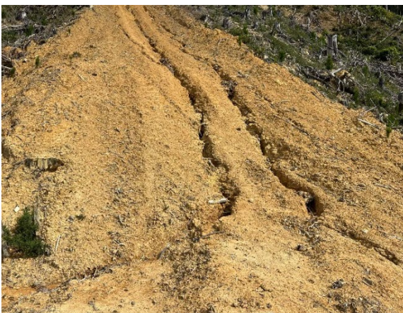
Figure 4: Lack of water controls.
