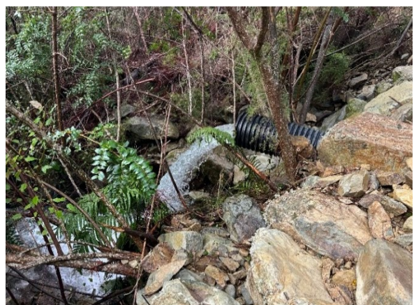
Figure 5: Perched Culvert and lack of fish passage.
